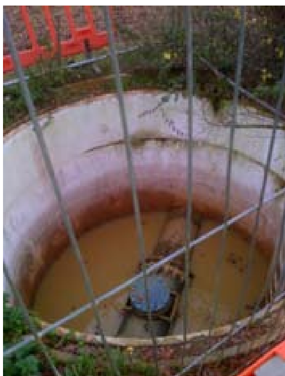
Figure 90: Showing the Rising Main manhole at the southern end of the site (RM3).
