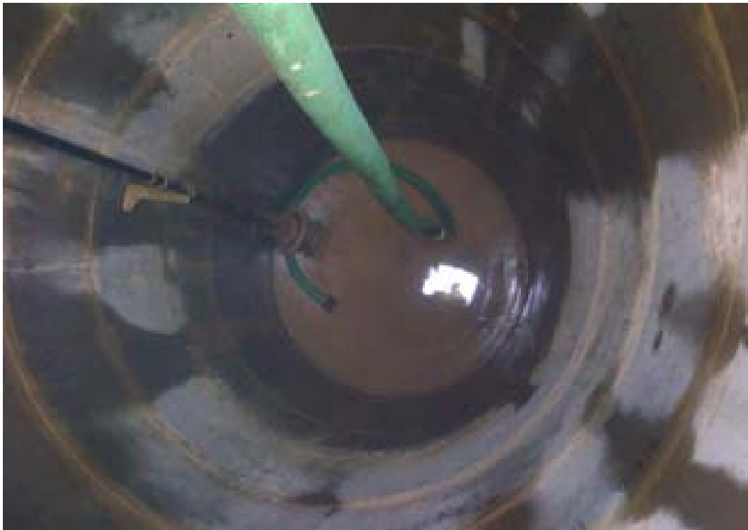
Figure 89: Showing the 7.5m deep Rising Main manhole at the northern end of the site adjacent to the canal (RM1).
