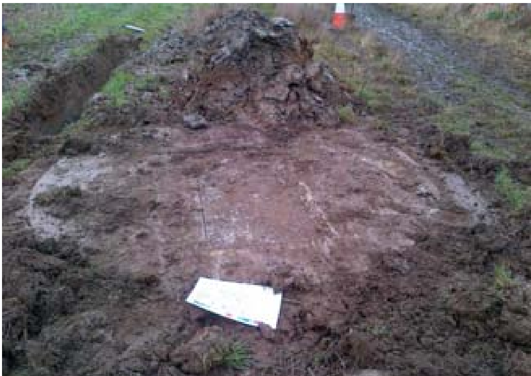
Figure 88: Showing the Rising Main manhole at the northern end of the site adjacent to the canal (RM1).
