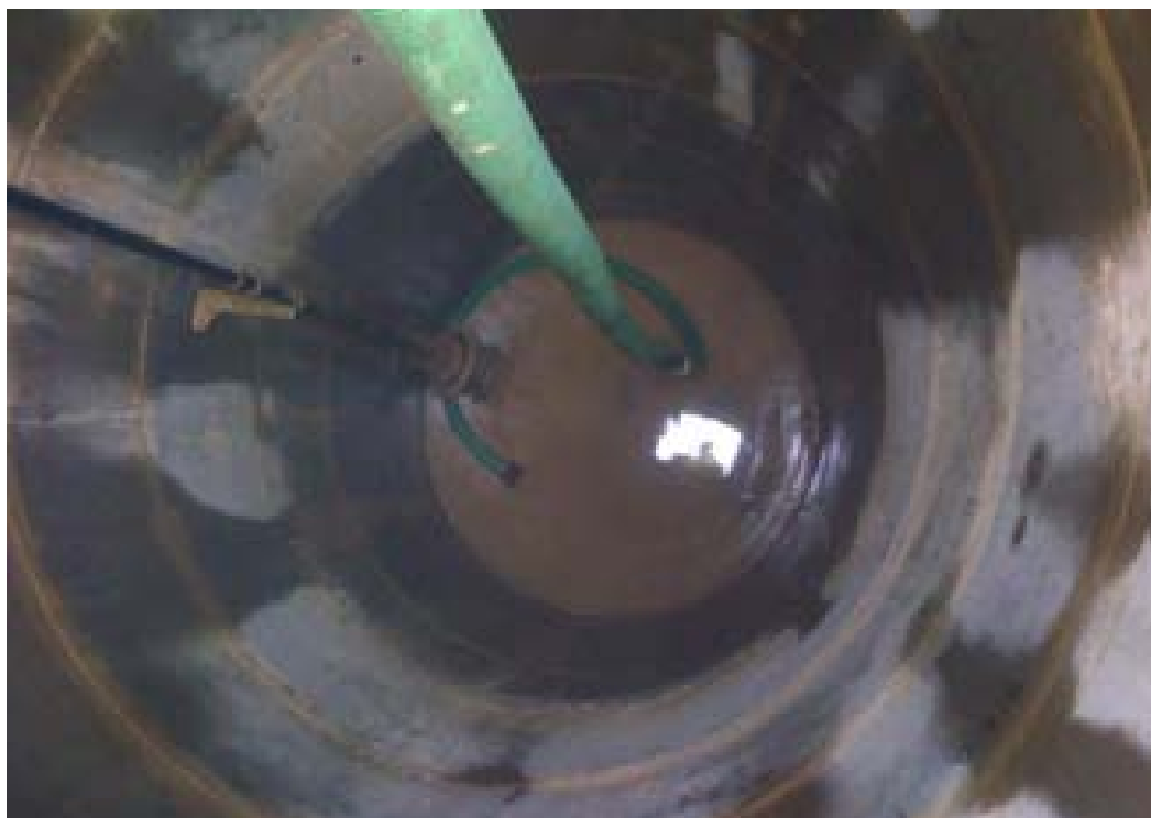
Figure 89: Showing the 7.5m deep Rising Main manhole at the northern end of the site adjacent to the canal (RM1).
