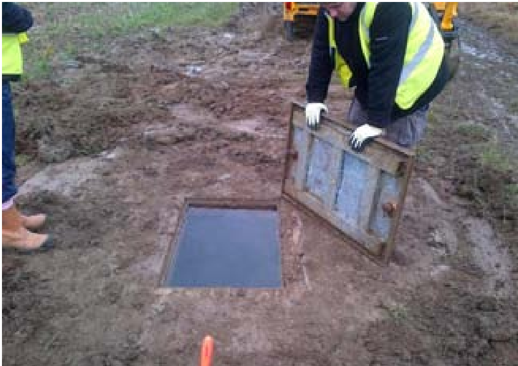
Figure 87: Showing the Rising Main manhole at the northern end of the site adjacent to the canal.
