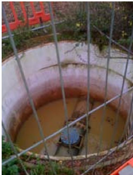
Figure 90: Showing the Rising Main manhole at the southern end of the site (RM3).
