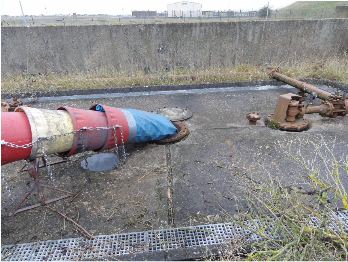
Photograph 384: POL tank chute filling
