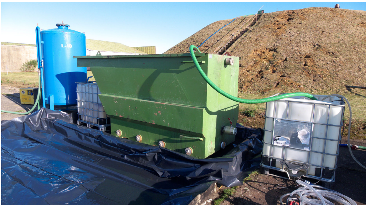
Photograph 367: Water treatment plant - POL22
