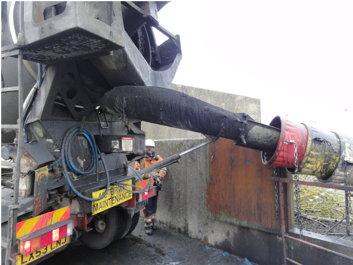
Photograph 381: POL tank chute filling
