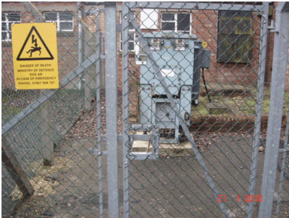
Plate 19: Distribution Substation DSS AR located adjacent to A1
