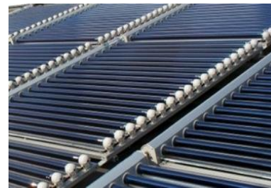
Figure 4.4: Solar Hot Water Panels
