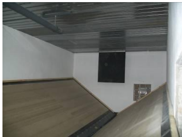
Figure 4.8: Example of biomass fuel storage: Internal masonry store
