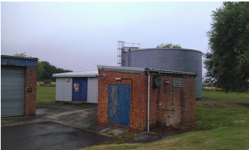
Foreground - Former diesel generator building to be retained. Brick garage building to be retained on LHS. Existing water tank and diesel pump house in background to be retained.
