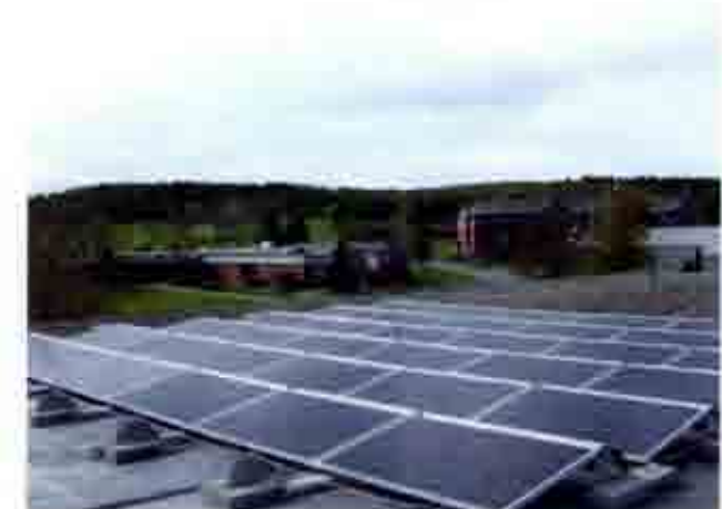
From the top: Solar thermal water heating, closed loop ground source heat pump and photovoltaic solar cells
