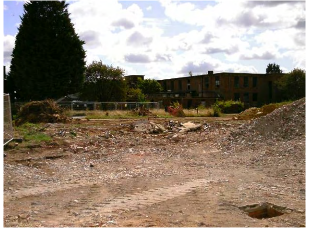
19.08.14 Centre of the site with building 498 that is to remain as part of the redevelopment
