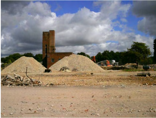
19.08.14 North-west corner of the site, boiler house (building 457) visible behind aggregate stockpile Agg-NW
