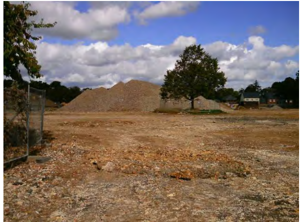
01.07.13 Northern view of Phase 1B: Area 1 with Aggregate Stockpile 'Agg-D1B-NE' in the background
