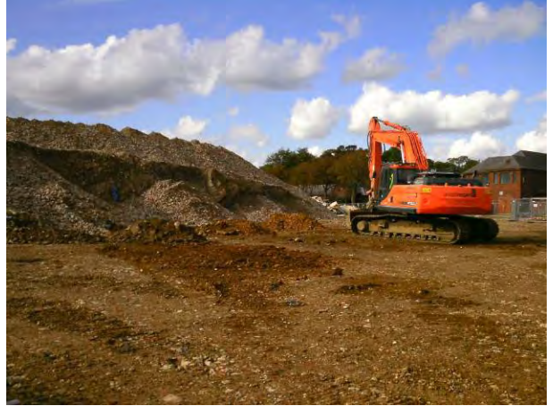
07.10.14 Excavation of entries to allow sampling around SS4 to delineate impacted soils
