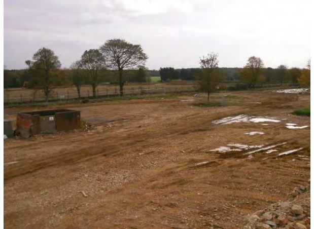
22.10.14 View to the south-east of the phase, substation visible in the left of the photo awaiting decommission and demolition at a later date
