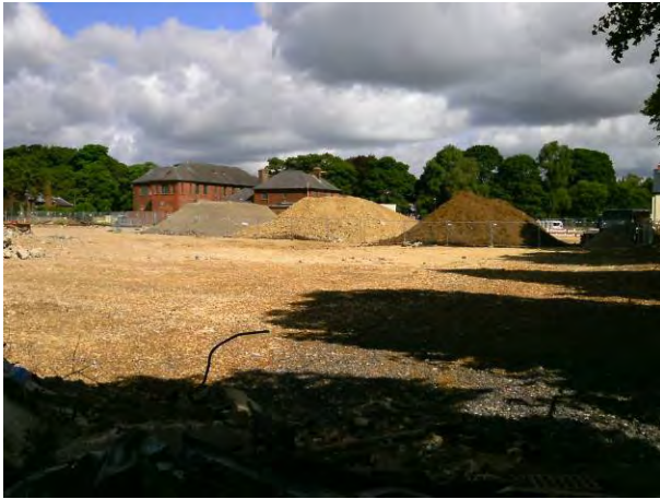
19.08.14 Northern end of the site following turnover and replacement of formation level strata
