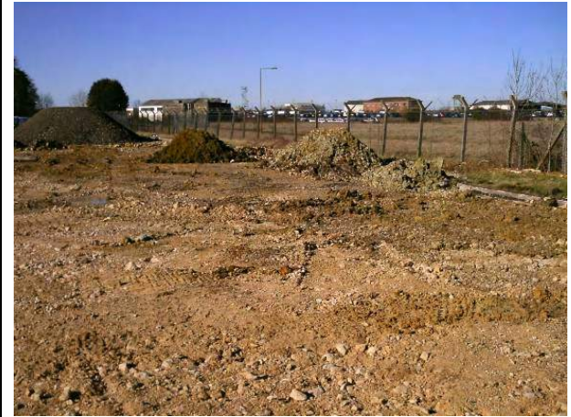
17.02.15 Trial-pits along the northern boundary confirming impacted soils extend off-site
