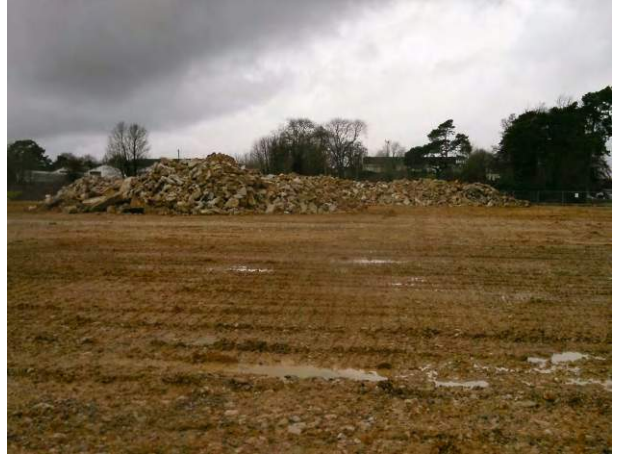
13.01.15 Stockpiles of site won hard-standing located in the centre and parallel to the western boundary awaiting processing
