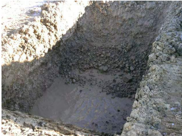
19.01.15 Excavation of trench 1 to determine location of removed soils (represented by MOT in-fill)
