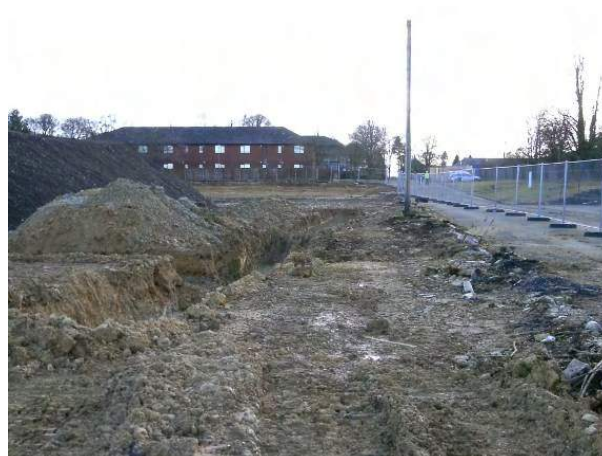
17.02.15 Trench in location of Jomas TP-NSA-231 reporting elevated hydrocarbons
