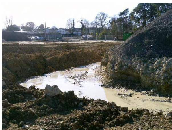
10.03.15 – Minor ingress of groundwater at bedrock level, no sheen observed
