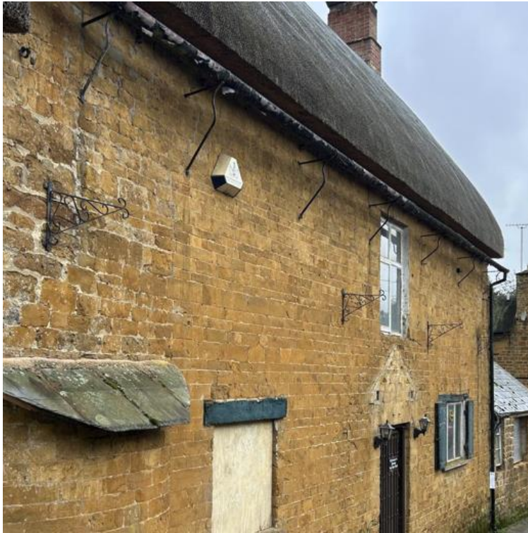
GUTTERS DOWNPIPES & BRACKETS
