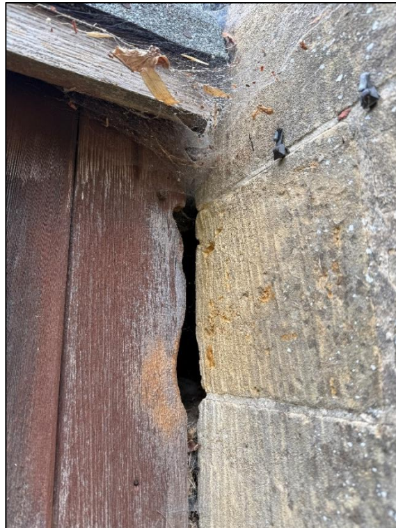
Plate 7. Gap between garage and house
