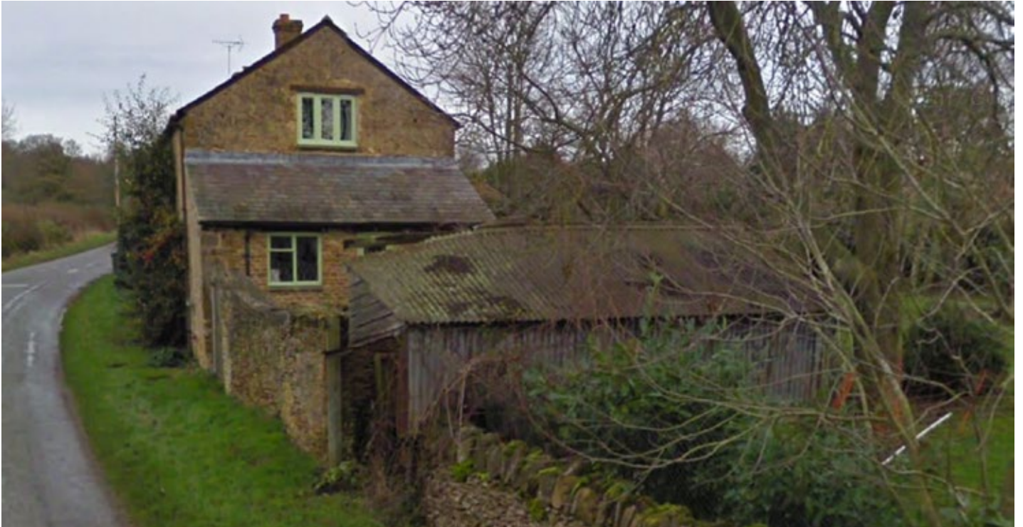
Street View image December 2009 of the former log store to the west of the cottage in dilapidated condition
