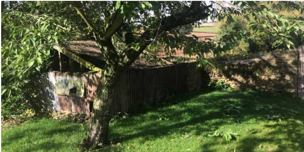
View of the dilapidated log store
