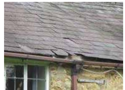
Damaged and slipped slate tiles
