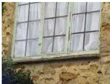
Existing North West Elevation - general state of windows
