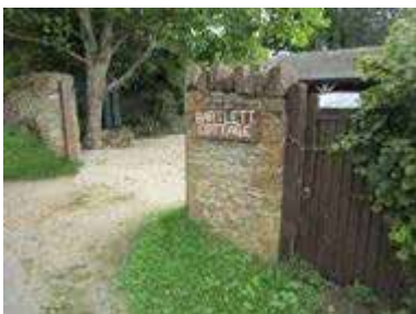
Existing pedestrian gate and missing vehicle gate
