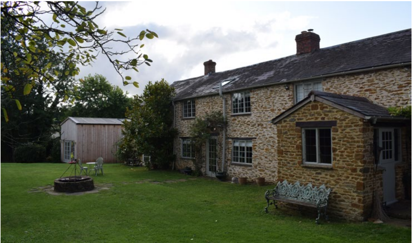
View of the rear (south) elevation with small porch and similar three-light casement windows, and Velux roof light.
