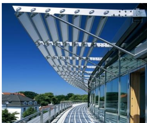
Figure 3 - Solar PV Louvres on the South Facade
