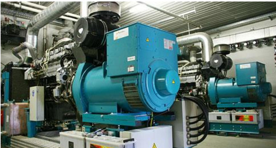
Figure 13 - Schnell Dual-Fuel Biomass CHP System
