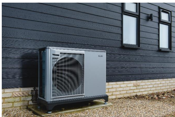
Figure 10 - Air Source Heat Pump
