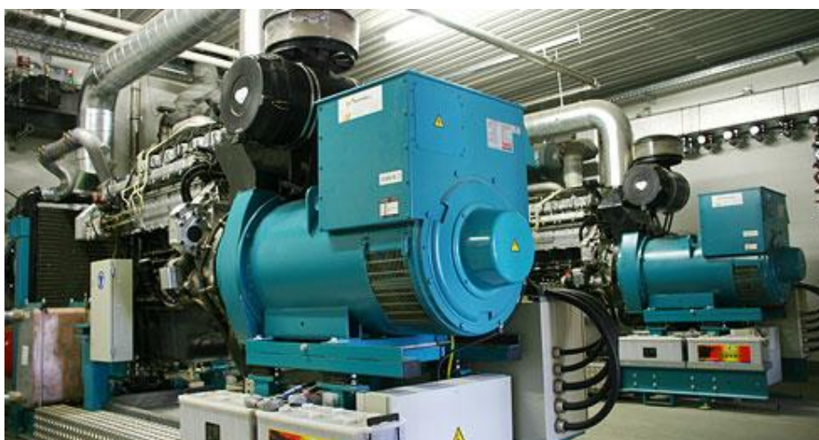
Figure 13 - Schnell Dual-Fuel Biomass CHP System
