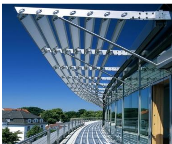
Figure 3 - Solar PV Louvres on the South Facade
