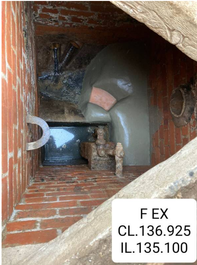
S106 Foul Connection
