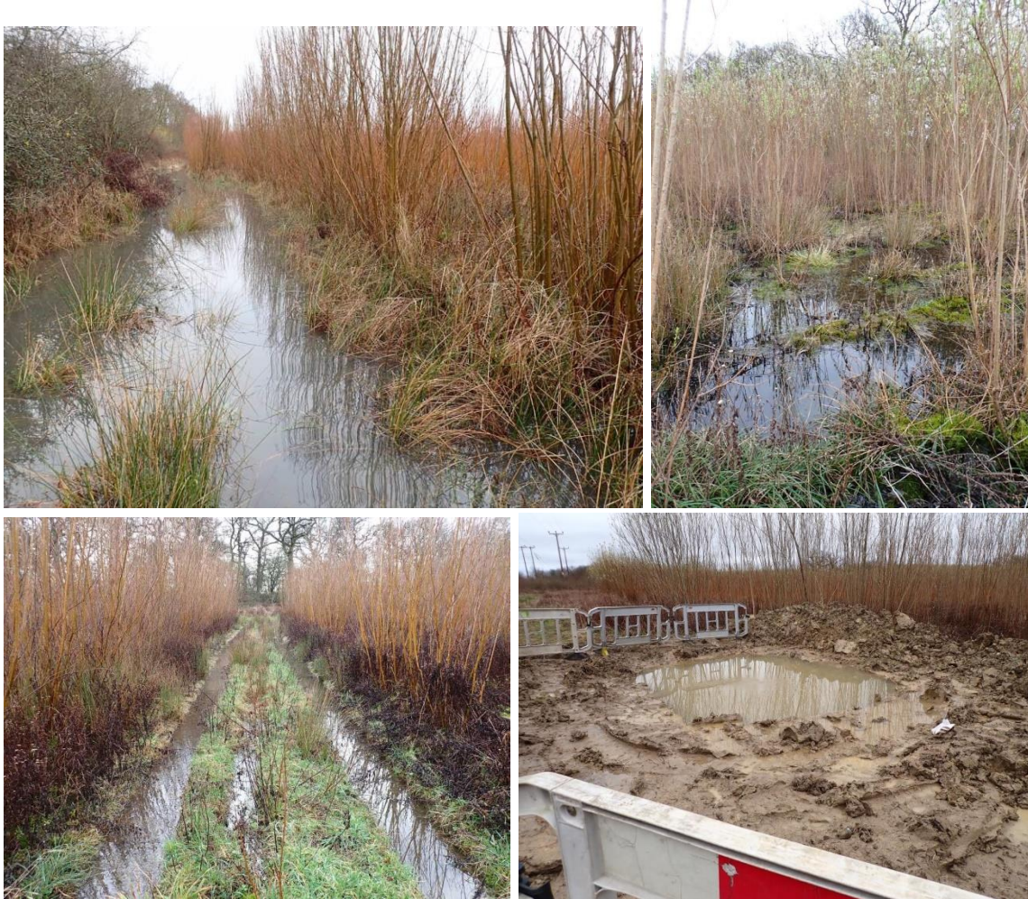
Winter flooding of the site, photographs from 02.01.2024 to 17.02.2024. Last photo shows how flooding is making leaking gas main repair by SGN very difficult
