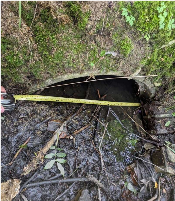
Figure A.9: Existing silted culvert
