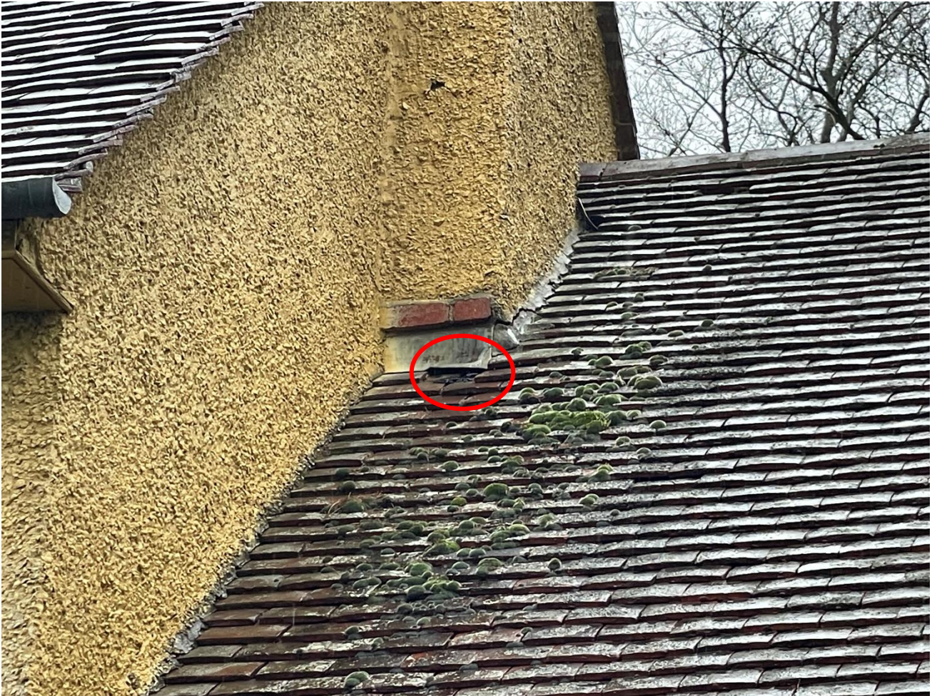
Figure 2. Missing tile below the eastern chimney stack of the dwelling (circled in red).
