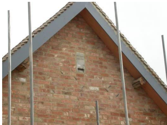
Fig. 7 Bat tube installed in gable end
