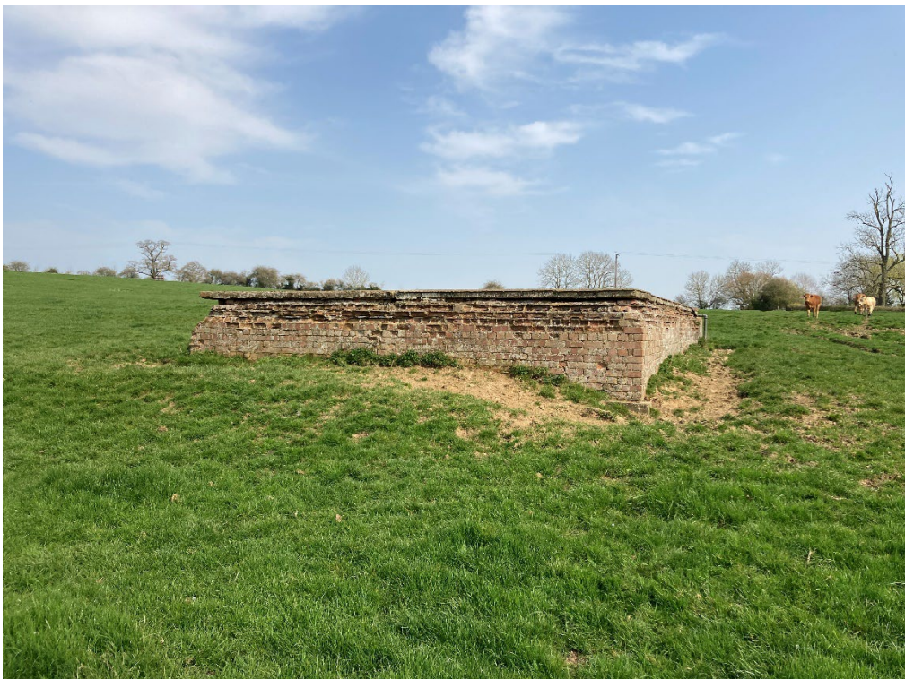
Photograph 6 - Relict structures considered to relate to a former water tank in the easternmost field
