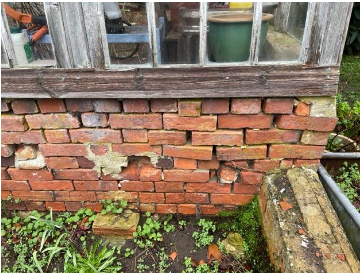
9 Derelict Horticultural Glass House
