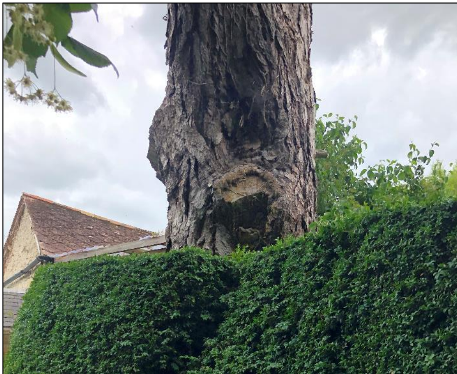
Figure 19: Rot hole at T1's south facing elevation
