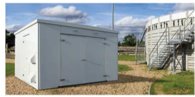
Indicative transformer enclosures
