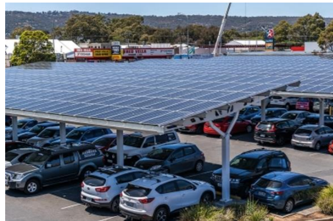
Figure 7: Solar PV car park canopies
