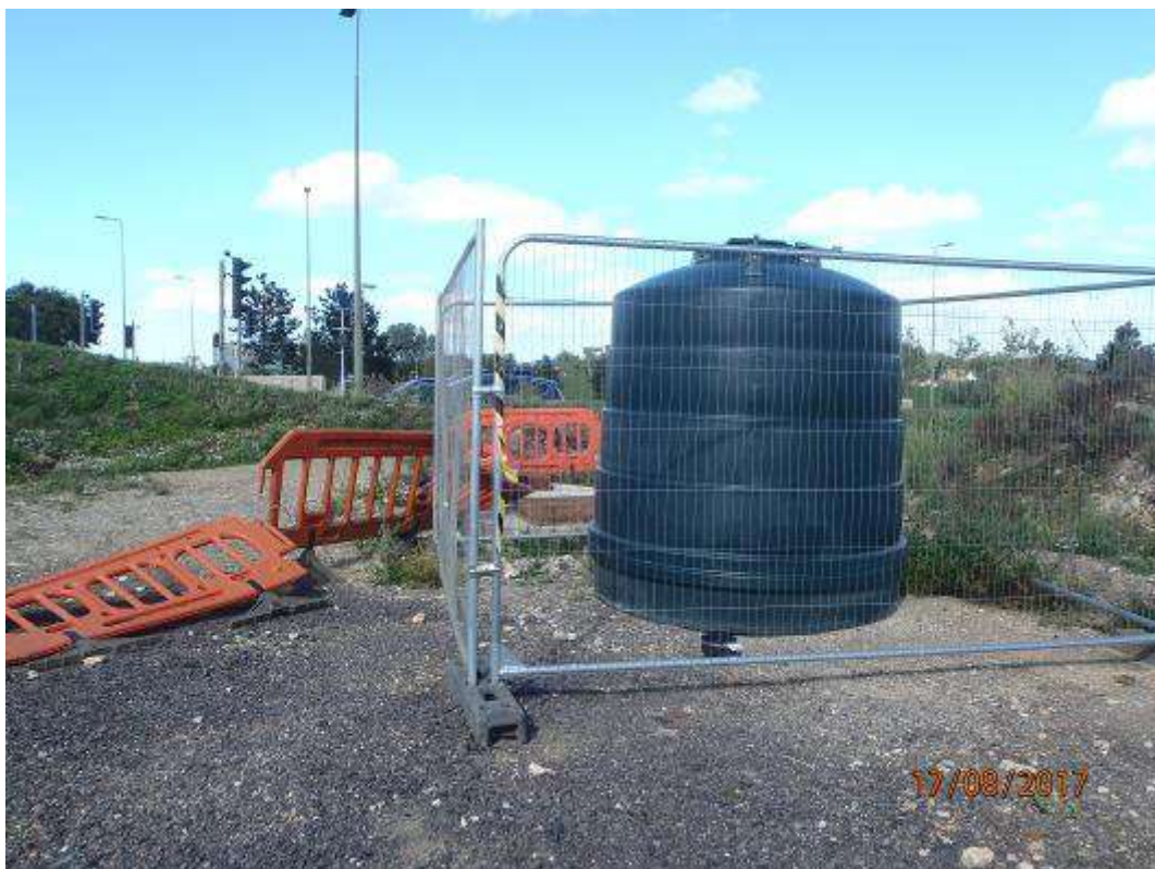
Photo 4— Water AST located along the boundary with Lakeview Drive.
