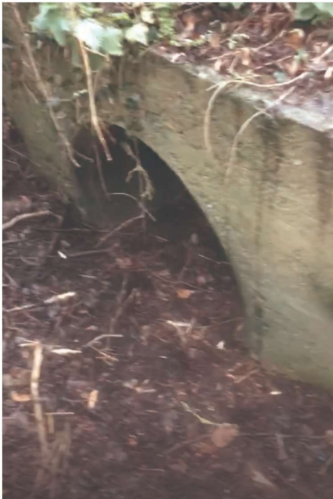
Figure 2.1: Culvert assumed to convey water from the western to eastern ditch along Yarnton/Green Lane
