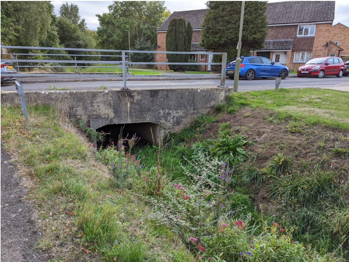
Figure 16.2: Ditch culverted under a road on site (photo taken during second site visit)
