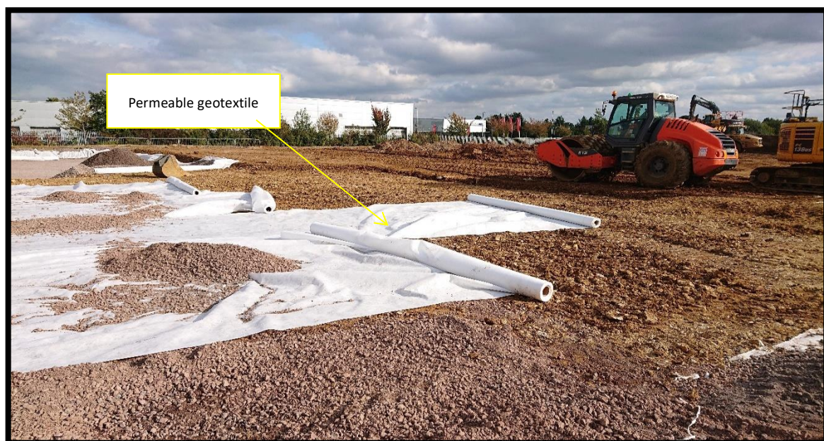
Fig 3.3.2- Image of geotextile being rolled out in preparation for the OGCR subbase.
