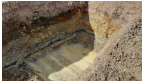
23.03.23 – Cell 12: Excavation progressed westwards with contaminated soils removed down to clean clays; significant contamination indicators absent along western sidewall but still present in southern sidewall (unable to progress due to standoff from Camp Road / live services).
