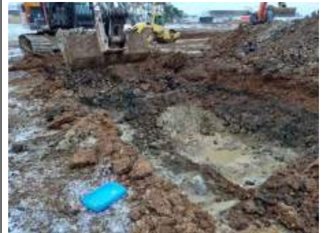
13.12.22 – Cell 8: Contaminated soils to west of Cell 4 excavated down to clean clays
