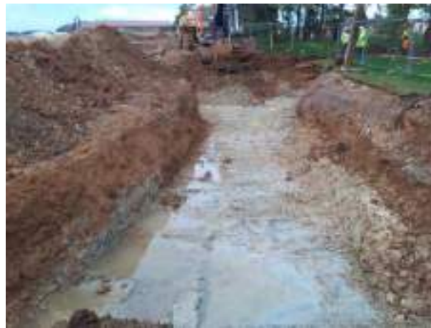
05.12.22 – Cell 3: Excavation progressed northwards with contaminated soils removed down to clean clays; contamination indicators absent along eastern sidewall.
