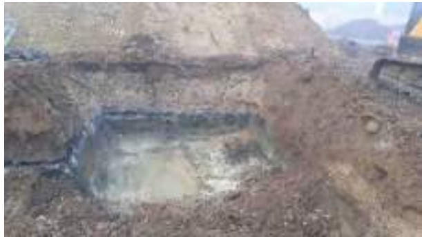
25.01.23 – Impacted soils removed with no significant contamination indicators at base or along eastern sidewall; thin band of impacted soils in northern sidewall but excavation constrained by presence of stockpile.
