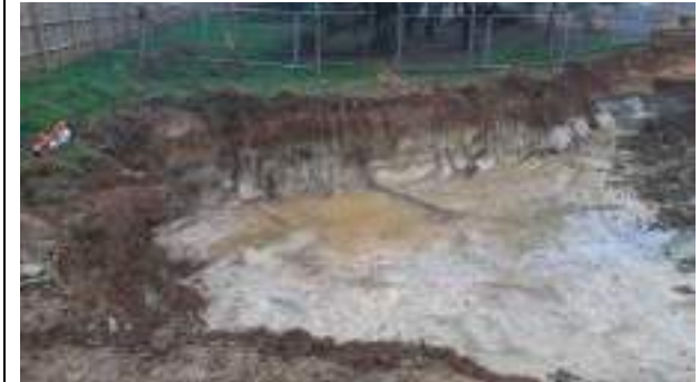
30.11.22 – Cell 2: Excavation progressed northwards and eastwards with contaminated soils removed down to clean clays; contamination indicators still present along western sidewall.
