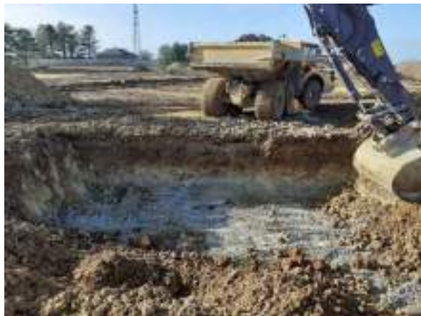
31.01.23 – Cell 2: Excavation progressed northwards with contaminated soils removed down to bedrock; significant contamination indicators absent along western sidewall.
