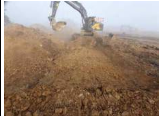
08.02.23 – Cell 6: Commencement of excavation along eastern extent of Cell 5; clean overburden soils placed into Cell 5 excavation area.
