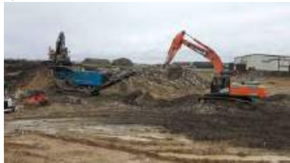
11.01.23 – Crushing of site-recovered hard materials to produce aggregate for reuse on site.
