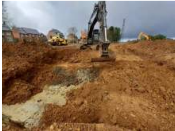
20.03.23 – Cell 10: Excavation progressed southwards (joining northern extent of Cell 9) and westwards with contaminated soils removed down to clean clays and clean overburden soils replaced into excavation area.
