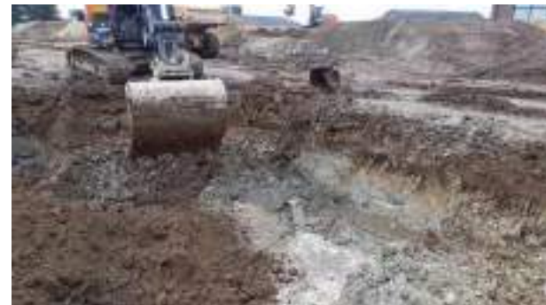
02.02.23 – Excavation continued along northern extent until significant contamination indicators were no longer present along northern sidewall (1/2).
