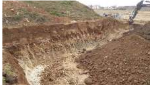
28.02.23 – View along eastern extent of NHS excavation; contamination indicators largely absent from sidewall with exception of in the approximate centre however these were present at depth (>2m bgl) and were located within a future POS area so further removal was not considered necessary.
