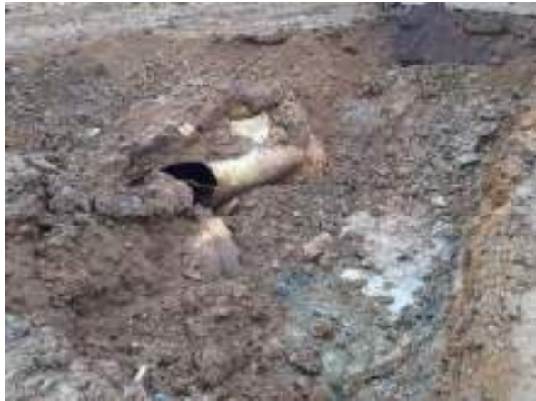
25.01.23 – Relict fibreglass interceptor encountered in centre-northwest of site underlain by black gravel and silver clays with strong hydrocarbon odours.
