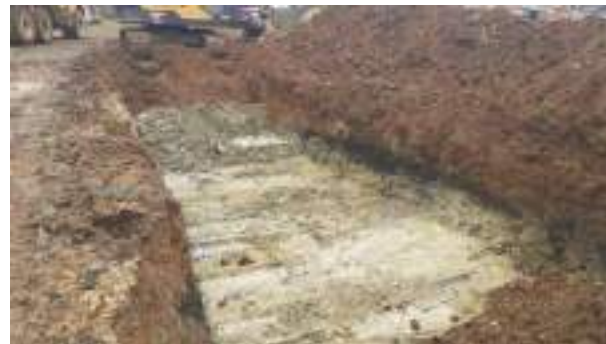
16.03.23 – Cell 9: Excavation progressed westwards with contaminated soils removed down to clean clays.
