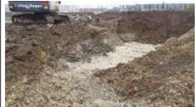
08.03.23 – Excavation progressed eastwards until joining with previously excavated / replaced soils; contaminated soils removed down to bedrock and clean overburden soils replaced into excavation; contamination indicators present along northern sidewall.
