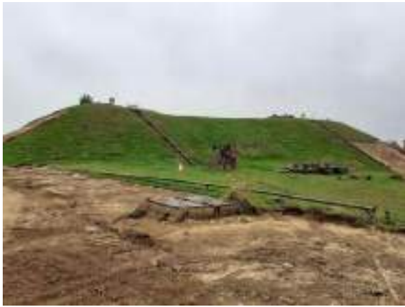
18.10.22 – Bund surrounding POL21 tanks in south of site.
