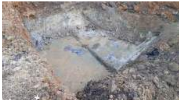
08.12.22 – Cell 6: Excavation of Cell 6 Hotspot complete; significant contamination indicators absent from base and sidewalls (1/2).
