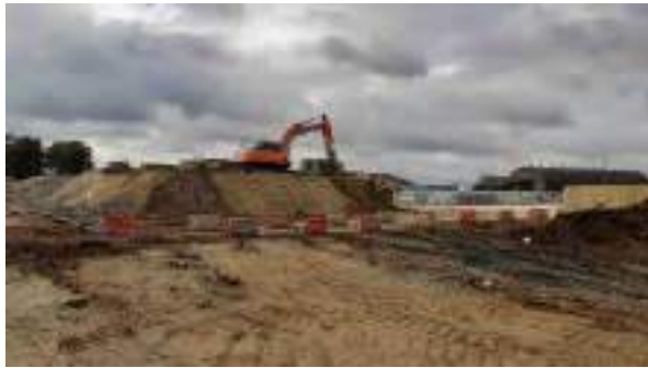
28.02.23 – Removal of contaminated soils to holding area within wider Heyford development site.
