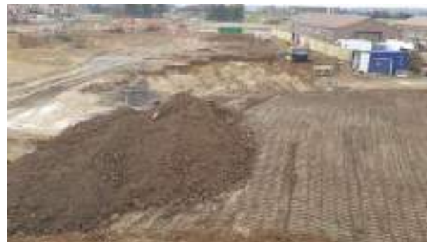
07.03.23 – Photograph showing southern and western extents of the western NHS excavation area prior to the final dig to north; topsoil earmarked for future POS areas stockpiled in eastern NHS excavation area (foreground).
