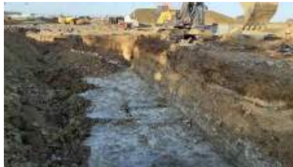
09.02.23 – Cell 7: Excavation progressed northwards with contaminated soils removed down to bedrock; significant contamination indicators absent along eastern sidewall.
