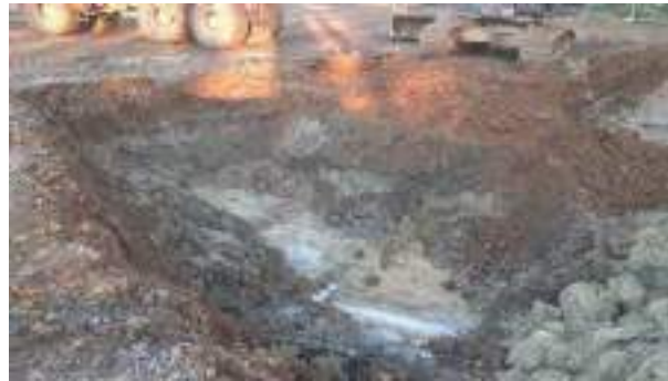
08.12.22 – Cell 7: Soils demonstrating slight contamination indicators but not significant enough to warrant removal so excavated, aerated and replaced into excavation.
