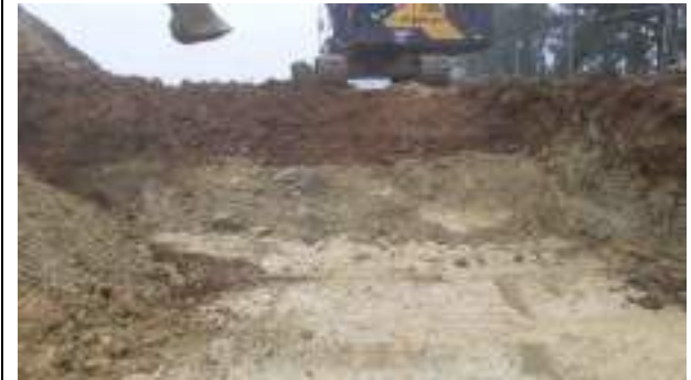
01.12.22 – Cell 2: Excavation progressed northwards with contaminated soils removed down to clean clays; contamination indicators absent along eastern part of northern sidewall.
