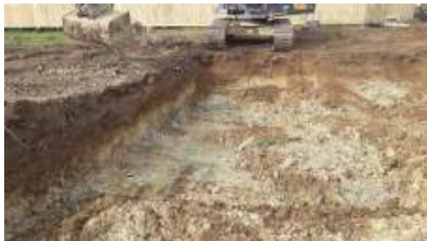
07.03.23 – Excavation continued to west; significant indicators of contamination absent along western and northern sidewalls and clay at base.
