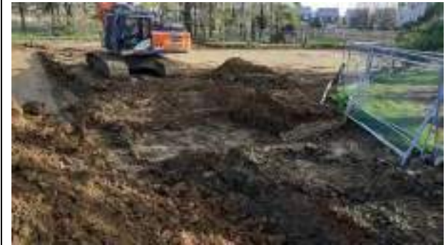
07.12.22 – Cell 5: Excavation continued to south of previous excavation area bridging gap to Cell1.
