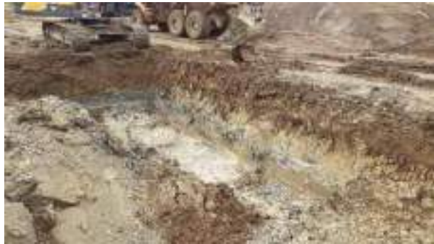
02.02.23 – Excavation continued along northern extent until significant contamination indicators were no longer present along northern sidewall (2/2).
