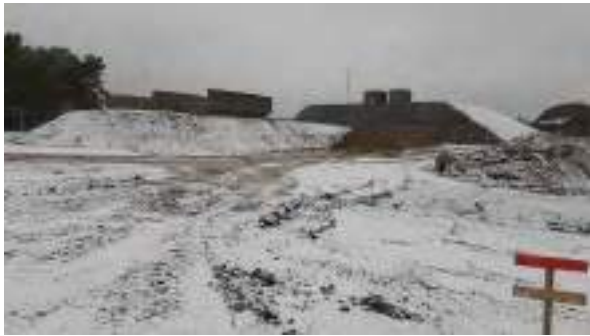
12.12.22 – Stockpiles of hydrocarbon contaminated soils located on hardstanding in the northwest of site.
