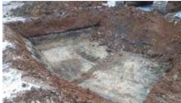
12.12.22 – Cell 7: Excavation continued to north of western part of previous excavation area; soils demonstrating slight contamination indicators but not significant enough to warrant removal so excavated, aerated and replaced into excavation.
