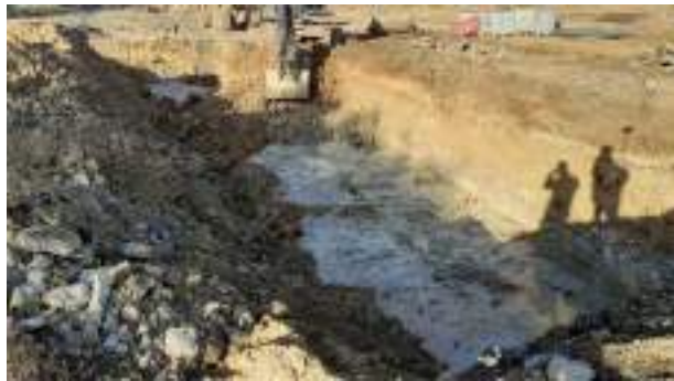
09.02.23 – Cell 7: Commencement of excavation along eastern extent of Cell 6; contaminated soils removed down to bedrock and clean overburden soils placed into Cell 6 excavation area.
