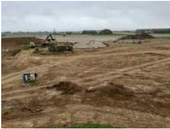
18.10.22 – View north across central area of site from south; topsoil strip carried out prior to site visit.
