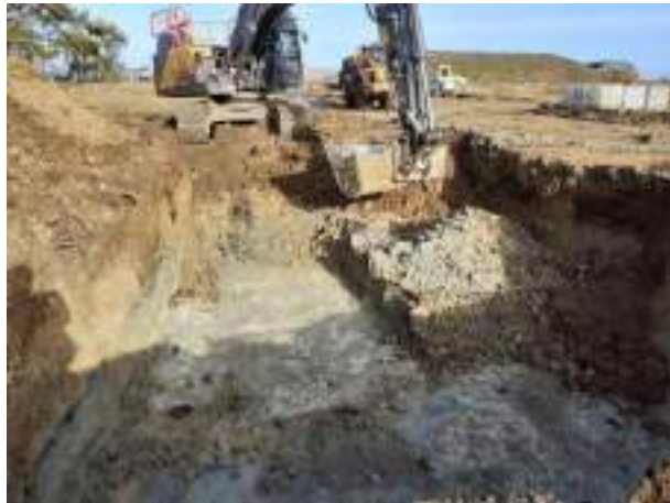
30.01.23 – Cell 2: Excavation commenced from southeast corner of Cell progressing north towards Cell 1 with contaminated soils removed down to bedrock; contamination indicators still present along eastern and western sidewalls.
