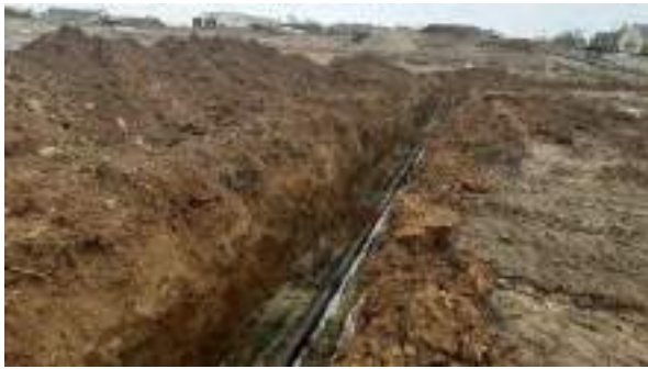
15.03.23 – POL pipeline uncovered in southwest of site demonstrating evidence of leakage – see hotspot records for further photos showing contamination removal.
