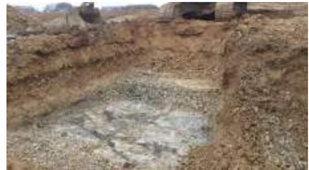
01.03.23 – Northeast corner of SHS excavation area; contaminated soils removed down to bedrock; no significant contamination indicators present along eastern or northern sidewalls with exception of the weathered bedrock at ~1.8-2.3m bgl.
