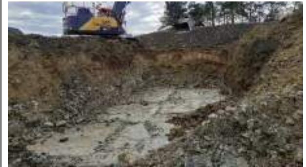
10.02.23 – Cell 7: Excavation progressed southwards with contaminated soils removed down to bedrock; significant contamination indicators absent along eastern, western and southern sidewalls.
