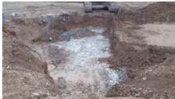
21.02.23 – Excavation progressed southwards alongside access road which curves to the east with contaminated soils removed down to bedrock and clean overburden soils replaced into excavation area; contaminated soils continued beneath roadway (2/2).
