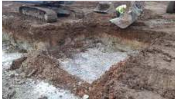
01.02.23 – Cell 3: Excavation progressed westwards from northern part of excavation area with contaminated soils removed down to bedrock; significant contamination indicators absent along western and southern sidewalls.
