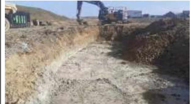
15.02.23 – Cell 8: Excavation progressed northwards / eastwards with contaminated soils removed down to bedrock and clean overburden soils placed into previous excavation area; significant contamination indicators absent along eastern sidewall.
