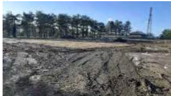
19.01.22 – Clean, recovered soils placed to raise levels in 'SW-HS' area prior to site visit.
