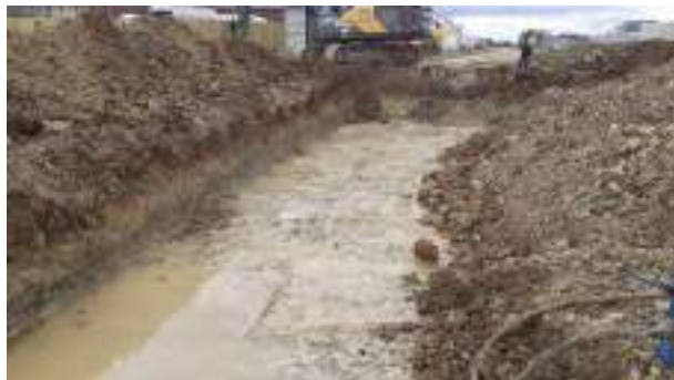
06.03.23 – Excavation progressed northwards with contaminated soils removed down to bedrock and clean overburden soils replaced into excavation; contaminated soils still present along northern / western sidewalls.
