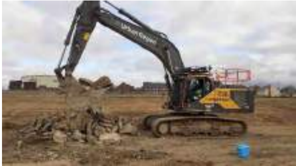
28.02.23 – Removal of site-recovered concrete to holding area within wider Heyford development site.
