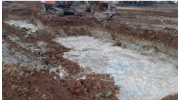
01.02.23 – Cell 3: Excavation progressed southwards with contaminated soils removed down to bedrock; significant contamination indicators absent along southern part of western sidewall and southern sidewall.
