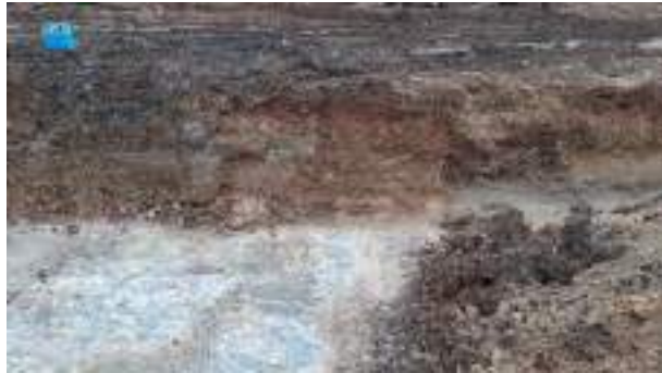
27.01.23 – Cell 1: Contamination appeared to be associated with a relict drain at interface between bedrock and superficial soils along eastern sidewall where the highest PID readings and strongest odours were noted.
