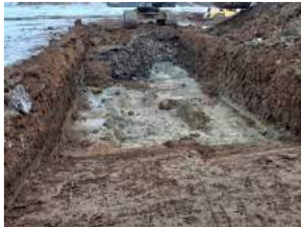
13.12.22 – Cell 8: Commencement of excavation to west of Cells 4-6; contamination indicators identified to west of Cell 4.
