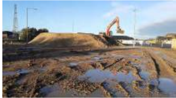
22.11.22 – Stockpile of hydrocarbon contaminated soils located on hardstanding in the northwest of site.
