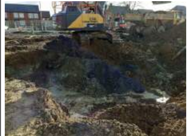
14.03.23 – Cell 9: Excavation progressed southwards alongside Cell 2 with contaminated soils removed down to clean clays
