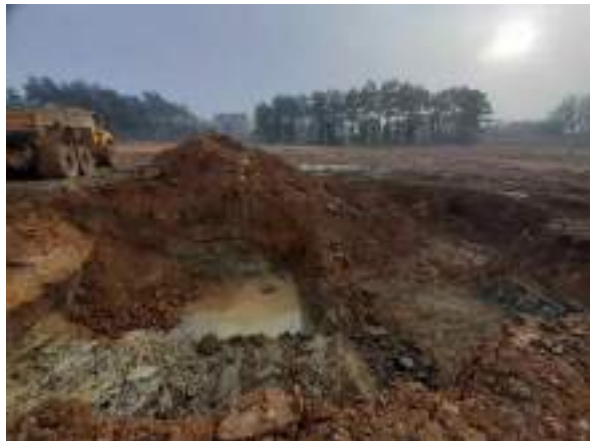
25.01.23 – Impacted soils in vicinity of interceptor removed; no significant contamination indicators at base or along southern or western sidewalls.
