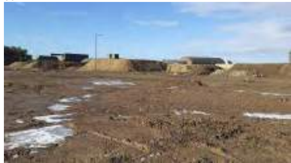
19.01.22 – Stockpiles of contaminated soils placed on concrete hardstanding along northern site boundary.
