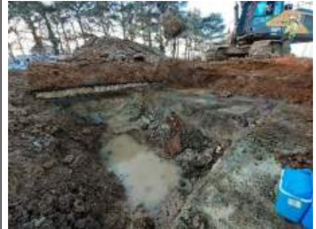
14.12.22 – Cell 8: Excavation progressed westwards with contaminated soils removed down to clean clays; significant contamination indicators absent along northern and southern sidewalls.
