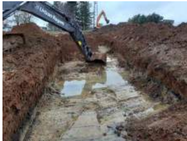
20.03.23 – Cell 10: Contaminated soils underlying, and to south of, former pipeline removed down to clean clays; significant contamination indicators absent from western sidewall but present in northern sidewall.
