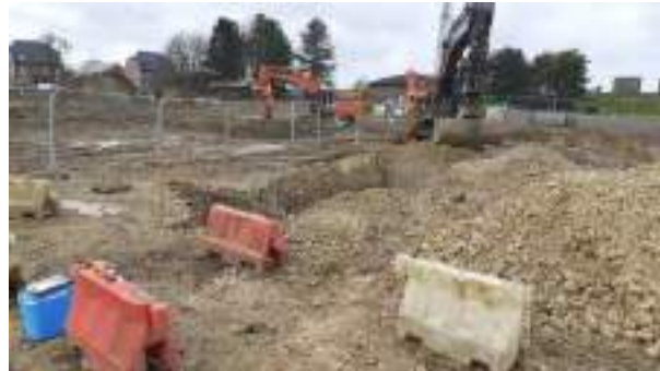
24.03.23 – View of hotspot area excavated over the previous day during backfilling with retained overburden soils.
