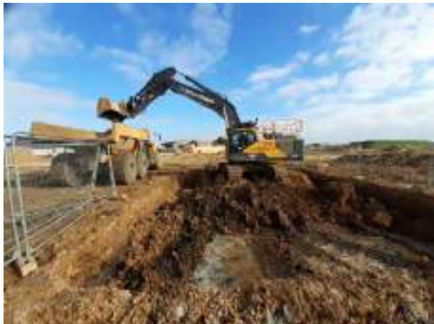
03.04.23 – Continuation of excavation with removal of ACM impacted soils to holding area.
