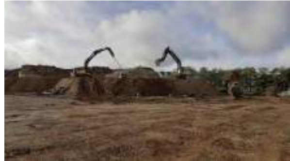
25.10.22 – Excavation and relocation of POL21 bund soils to expose upper extents of tanks.
