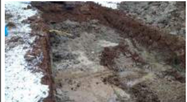
12.12.22 – Cell 7: Excavation of Cell 7 Hotspot progressed eastwards; contamination indicators absent from base and western / southern / eastern sidewalls but still present in northern sidewall (2/2).
