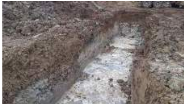
01.02.23 – Excavation continued southwards until significant contamination indicators were no longer present along southern sidewall.
