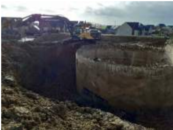
23.11.22 – Excavation of soils around POL21B tank to fully expose walls; soils demonstrating contamination indicators removed to contamination stockpiles in northwest
