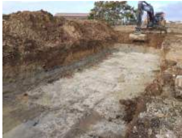
30.01.23 – Cell 2: Excavation progressed north towards Cell 1 with contaminated soils removed down to bedrock; contamination indicators still present along eastern and western sidewalls.
