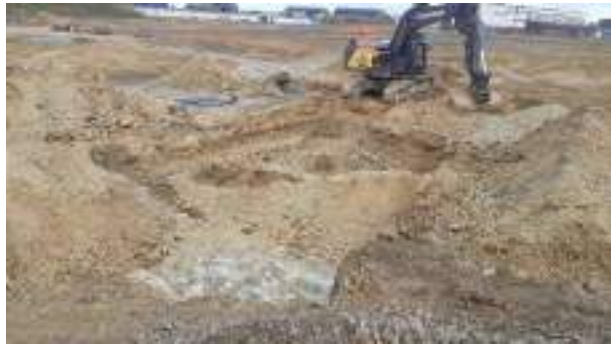
01.03.23 – View of entire SHS excavation area during backfilling with retained overburden soils.
