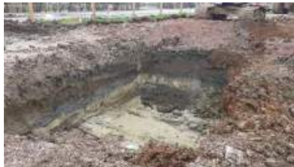
22.03.23 – Cell 12: Excavation progressed westwards with contaminated soils removed down to clean clays; contamination indicators present in southern sidewall but unable to progress due to standoff from Camp Road / live services.
