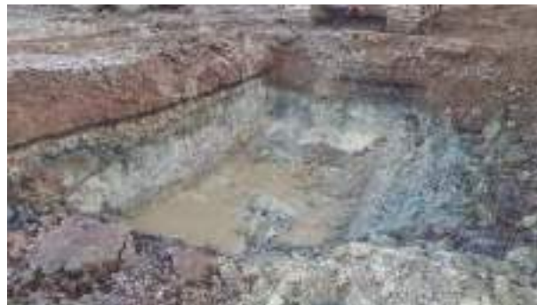
08.12.22 – Cell 6: Excavation of Cell 6 Hotspot complete; significant contamination indicators absent from base and sidewalls (2/2).
