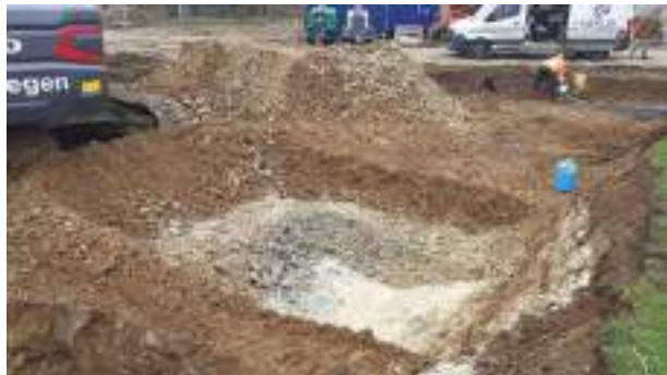
21.02.23 – Commencement of NHS hotspot excavation from northern site boundary / to east of site access road.
