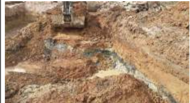
23.03.23 – Cell 12: Excavation progressed westwards with contaminated soils removed down to clean clays; contamination indicators still present in western / northern sidewalls however these were present at depth (>2m bgl) within a thin band of soils (circa. 0.5m thick) so deemed impractical to remove and considered unlikely to present a significant risk to human health and/or the environment.
