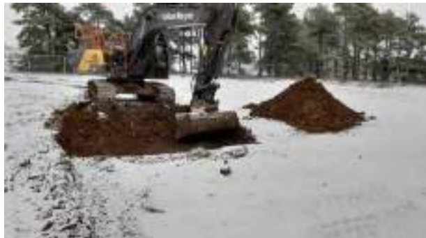
12.12.22 – Cell 7: Recommencement of excavation to east of previous excavation area; clean overburden soils side-cast.
