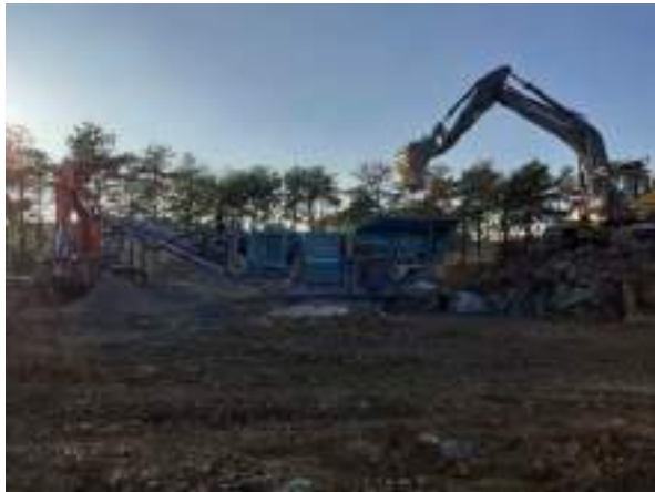
23.01.23 – Crushing of site-recovered hard materials to produce aggregate for reuse on site.
