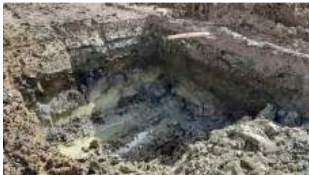
22.03.23 – Cell 12: Contaminated soils removed down to clean clays; significant contamination indicators absent from eastern sidewall.
