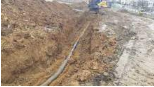
15.03.23 – Second POL pipeline uncovered in southwest of site – no evidence of leakage (2/2).
