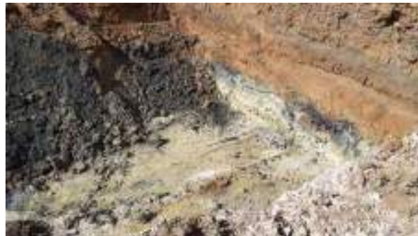
23.03.23 – Cell 12: Excavation progressed westwards with contaminated soils removed down to clean clays; contamination indicators still present in northern sidewall however these were present at depth (>2m bgl) within a thin band of soils (circa. 0.5m thick) so deemed impractical to remove and considered unlikely to present a significant risk to human health and/or the environment.
