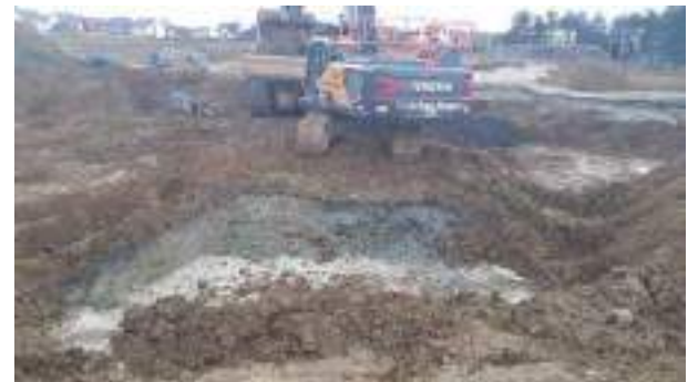
22.02.23 – Excavation continued to east of initial excavation area and progressed southwards; contaminated soils removed down to bedrock and clean overburden soils replaced into excavation area.
