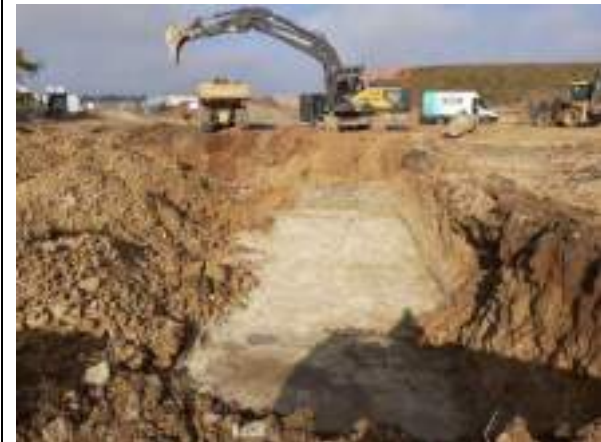
14.02.23 – Cell 8: Excavation progressed northwards with contaminated soils removed down to bedrock and clean overburden soils placed into Cell 2 excavation area; significant contamination indicators absent along eastern sidewall.
