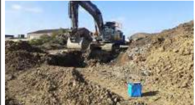
02.03.23 – Excavation continued to west of previous excavation area in footprint of former roadway.
