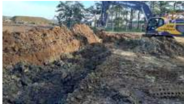
07.12.22 – Cell 5: Excavation and replacement of soils progressed eastwards to eastern extent of Cell 5.
