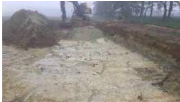
01.12.22 – Cell 2: Excavation progressed northwards and eastwards with contaminated soils removed down to clean clays; contamination indicators still present along eastern sidewall.
