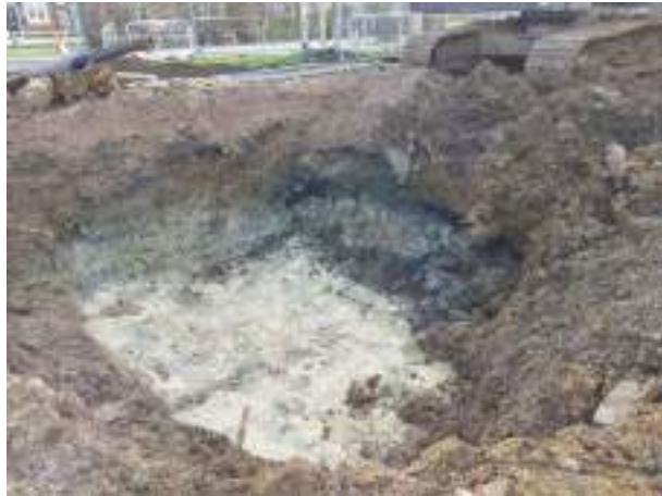
21.03.23 – Cell 11: Excavation progressed westwards; contamination indicators still present in southern and western sidewalls (unable to progress due to standoff from Camp Road / live services and live drain, respectively).
