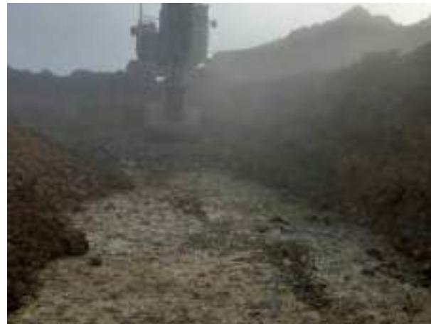
08.02.23 – Cell 5: Excavation progressed to south and east with contaminated soils removed down to bedrock; significant contamination indicators absent along southern sidewall but still present along eastern sidewall.
