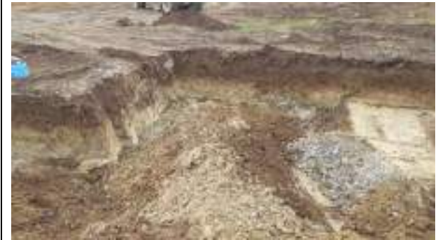
07.03.23 – Excavation continued to west; significant indicators of contamination absent along western sidewall (1/2).
