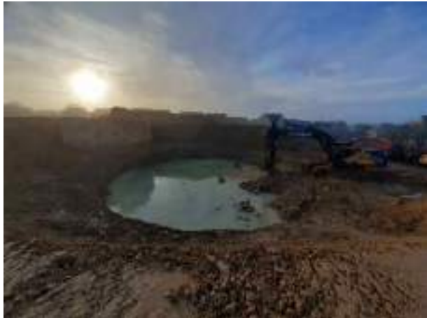
28.11.22 – Demolition of tank walls complete; clearance of demolition rubble from tank base.
