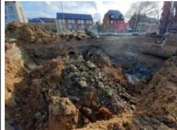
21.03.23 – Cell 11: Excavation progressed westwards; contamination indicators still present in southern sidewall (unable to progress due to standoff from Camp Road / live services).
