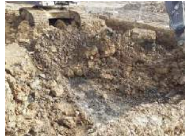
03.04.23 – Fragments of ACM identified in soils; impacted soils therefore excavated and transferred to holding area within wider Heyford Development site.
