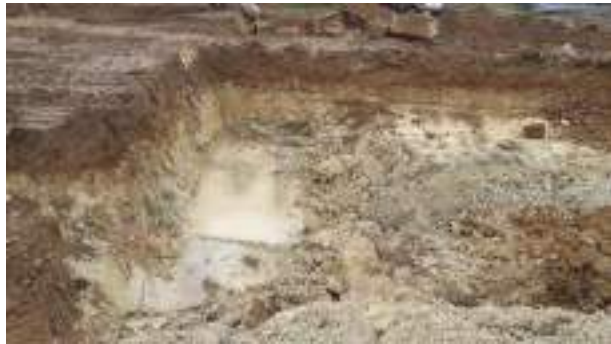
08.03.23 – Excavation progressed eastwards with contaminated soils removed down to clean clays and clean overburden soils replaced into excavation; significant contamination indicators absent along northern and western sidewalls.
