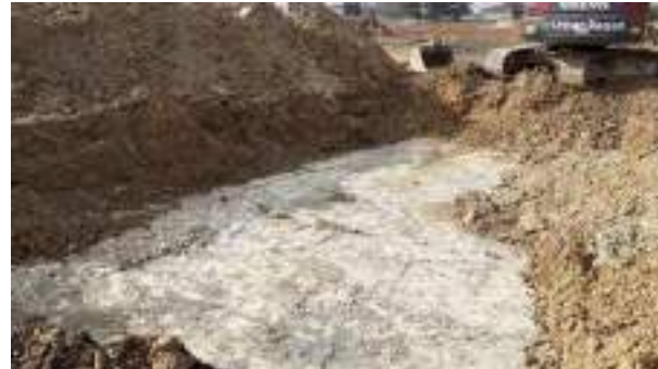
02.03.23 – Excavation progressed southwards to northern extent of CHS excavation area and westwards until contamination indicators were absent from sidewall; contaminated soils removed down to bedrock and clean overburden soils replaced into excavation.
