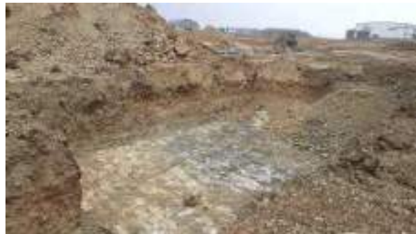
01.03.23 – Northern extent of SHS excavation area: contaminated soils removed down to bedrock; no significant contamination indicators present along northern sidewall.
