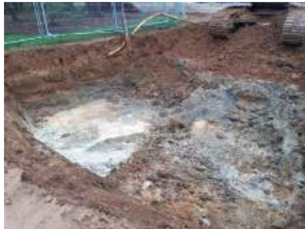
29.11.22 – Cell 1: Contaminated soils removed down to clean clays; contamination indicators still present along western sidewall.
