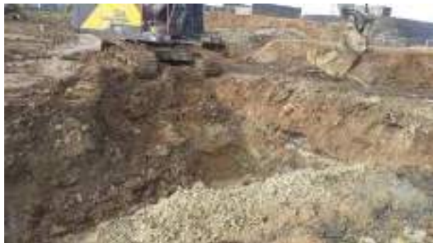
26.01.23 – Excavation of impacted soils progressed to west until significant contamination indicators absent from base and western sidewall.
