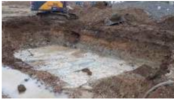
02.02.23 – Cell 4: Excavation progressed eastwards with contaminated soils removed down to bedrock; contamination indicators present along both eastern and southern sidewalls.
