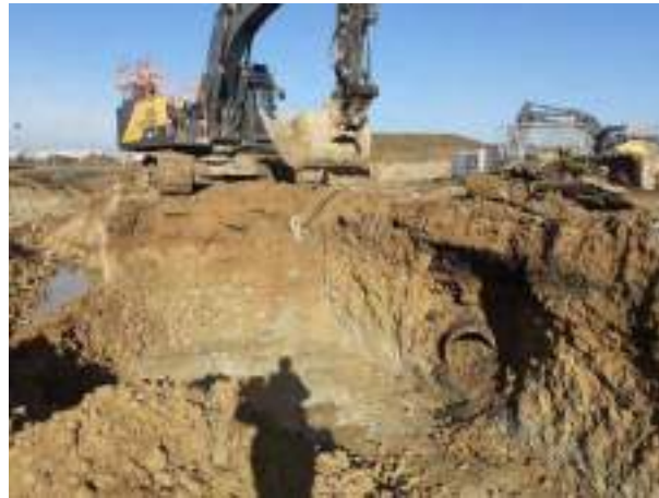
08.02.23 – Cell 6: Excavation progressed northwards with contaminated soils removed down to bedrock; contamination indicators still present along eastern sidewall.
