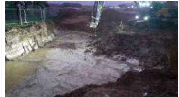
30.11.22 – Cell 2: Excavation progressed northwards (until joined with Cell 1) and eastwards with contaminated soils removed down to clean clays.
