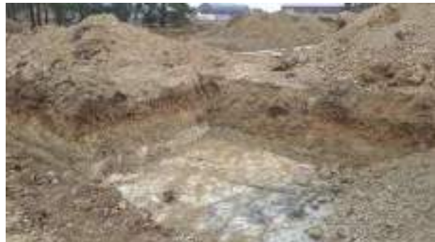
01.03.23 – Northwest corner of SHS excavation area: contaminated soils removed down to bedrock; no significant contamination indicators present along western or northern sidewalls.
