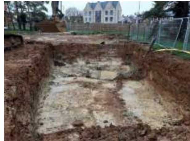
29.11.22 – Cell 1: Excavation progressed northwards with contaminated soils removed down to clean clays; contamination indicators still present along western sidewall.
