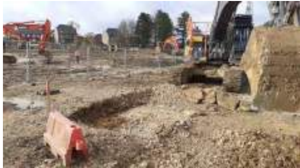
24.03.23 – Following removal of soil stockpile excavation progressed to north (red stake placed at northeast corner of previous excavation area).
