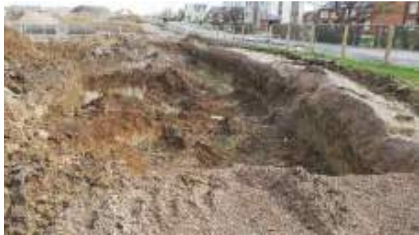
23.03.23 – Cell 12: View of entire Cell 12 excavation area; clean overburden soils replaced into excavation.
