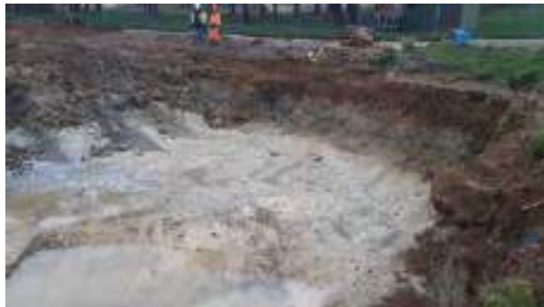
30.11.22 – Cell 2: Excavation progressed northwards and eastwards with contaminated soils removed down to clean clays; contamination indicators still present along eastern sidewall.
