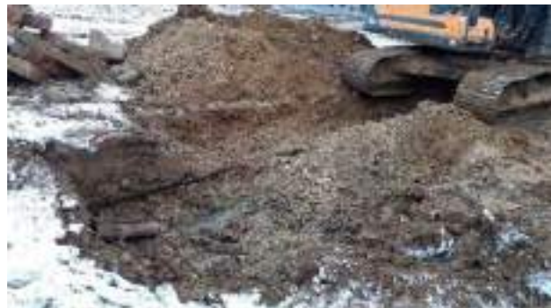
12.12.22 – Contaminated soils encountered in centre-north of site underlying relict pipeline.
