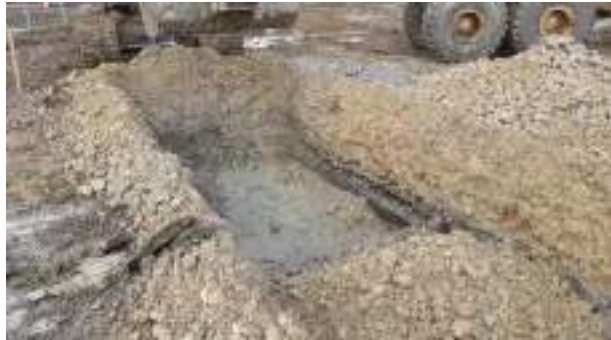
24.03.23 – Excavation progressed to west and thin band of contaminated gravel and clay removed; significant contamination indicators absent from base and western sidewall but still present along northern sidewall – not progressed any further as outside of proposed development area.
