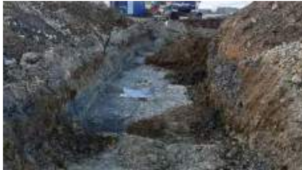
02.03.23 – Excavation progressed northwards along former roadway with contaminated soils removed down to bedrock; contaminated soils still present along northern / western sidewalls.
