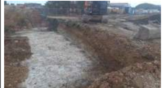
16.02.23 – Cell 8: Excavation of contaminated soils complete; significant contamination indicators absent along western and northern sidewalls.
