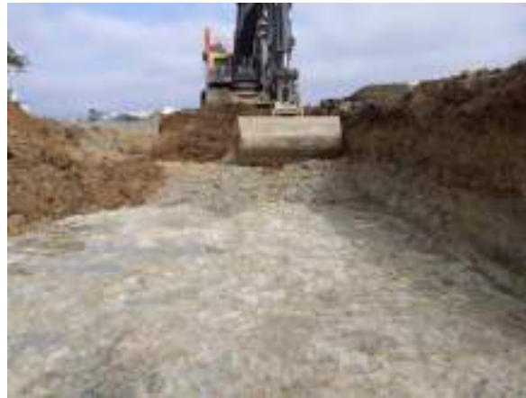
13.02.23 – Cell 8: Commencement of excavation from northern extent of Cell 7 / eastern extent of Cell 2.
