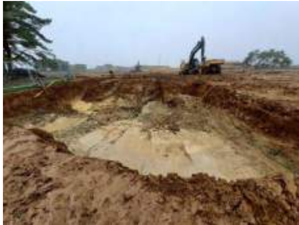
29.11.22 – Cell 1: Excavation progressed northwards with contaminated soils removed down to clean clays; contamination indicators still present along all four sidewalls.
