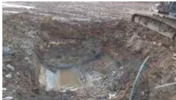
26.01.23 – Excavation of impacted soils progressed to west and south until significant contamination indicators absent from base and western and southern sidewalls (southwest corner of excavation area).
