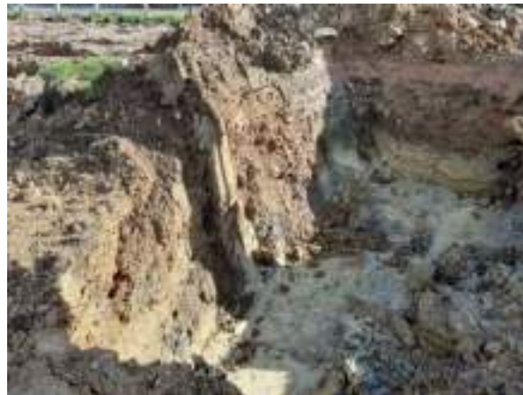
21.03.23 – Cell 11: Contaminated soils removed down to clean clays; significant contamination indicators absent from eastern sidewall but present in southern sidewall (unable to progress due to standoff from Camp Road / live services).
