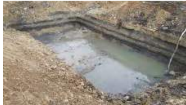
11.01.23 – POL2 (North) tanks removed and base and sidewalls exposed (partially limestone bedrock); view northeast.
