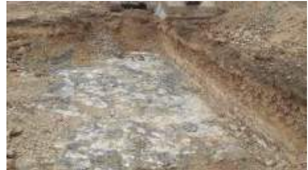
01.03.23 – Southern extent / southeast corner of SHS excavation area: contaminated soils removed down to bedrock; no significant contamination indicators present along eastern or southern sidewalls.
