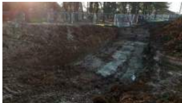
07.12.22 – Cell 5: Excavation and replacement of soils progressed eastwards to eastern extent of Cell 5.
