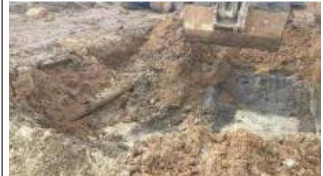
15.03.23 – Cell 9: Excavation continued to west of live drain / north of haul road; relict water main encountered alongside road which was removed.
