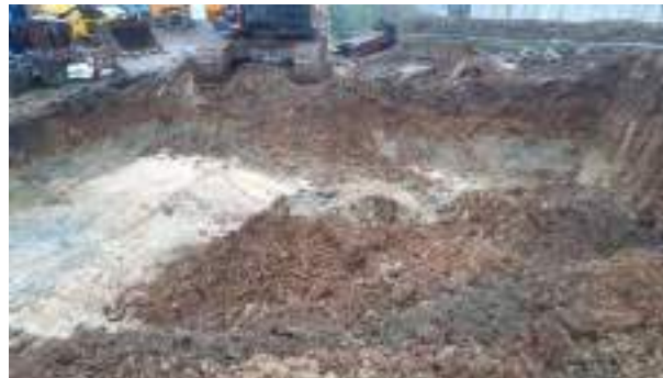
08.03.23 – Excavation progressed northwards / eastwards with contaminated soils removed down to bedrock and clean overburden soils replaced into excavation; thin band of potentially contaminated soil still present along northern sidewall from ~1.1m bgl however excavation nearing site boundary and any retained impacted soils will be located in future POS area.
