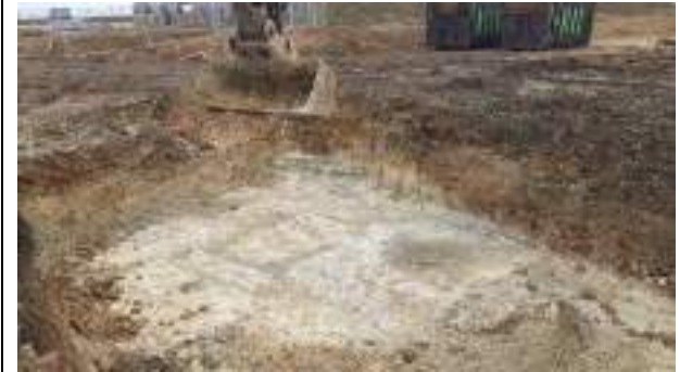
27.01.23 – Cell 1: Excavation progressed northwards with contaminated soils removed down to bedrock and clean overburden soils replaced into excavation; contamination indicators still present along eastern sidewall and eastern part of northern sidewall.
