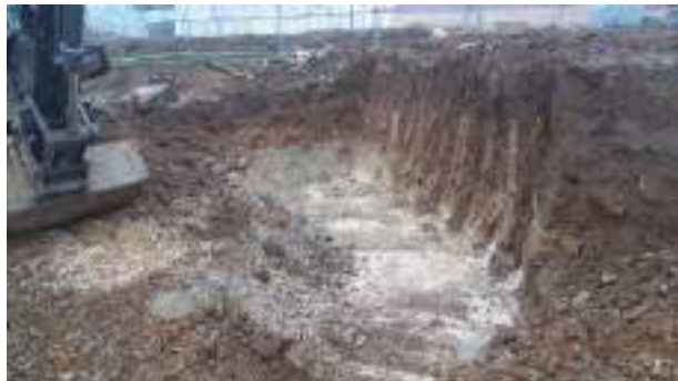
08.03.23 – Excavation progressed northwards with contaminated soils removed down to bedrock and clean overburden soils replaced into excavation; thin band of potentially contaminated soil still present along northern sidewall from ~1.1m bgl however excavation nearing site boundary and any retained impacted soils will be located in future POS area.
