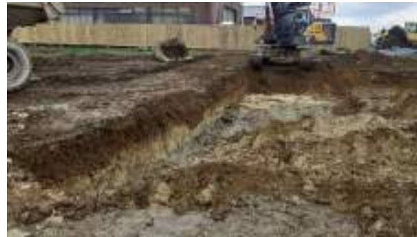
07.03.23 – Excavation progressed northwards with contaminated soils removed down to bedrock / clean clays and clean overburden soils replaced into excavation; contaminated soils still present along northern / western sidewalls.
