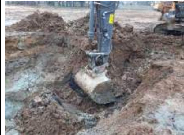
25.01.23 – Excavation and removal of hydrocarbon impacted soils in vicinity of former interceptor.
