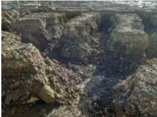
03.04.23 – Foundation excavation in area of Plots 1-2 in centre-northwest of site; drums infilled with concrete and posts identified amongst excavation.
