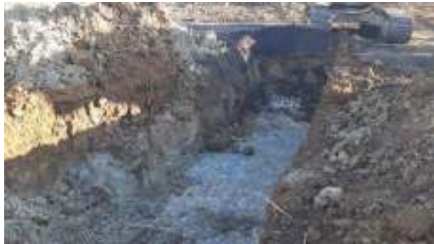
07.03.23 – Cell 9: Excavation progressed northwards with contaminated soils removed down to bedrock; significant contamination indicators absent along eastern sidewall.
