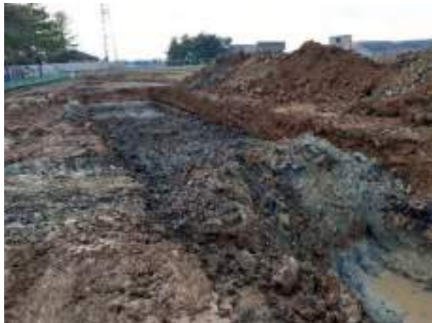
06.12.22 – Cell 4: Excavation and replacement of soils progressed eastwards to eastern extent of Cell 4.
