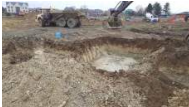
07.03.23 – Excavation continued to west; contamination indicators absent along southern part of western sidewall.
