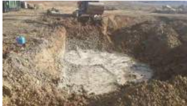
15.02.23 – Cell 8: Excavation progressed northwards / eastwards with contaminated soils removed down to bedrock and clean overburden soils placed into previous excavation area; significant contamination indicators absent along eastern sidewall.
