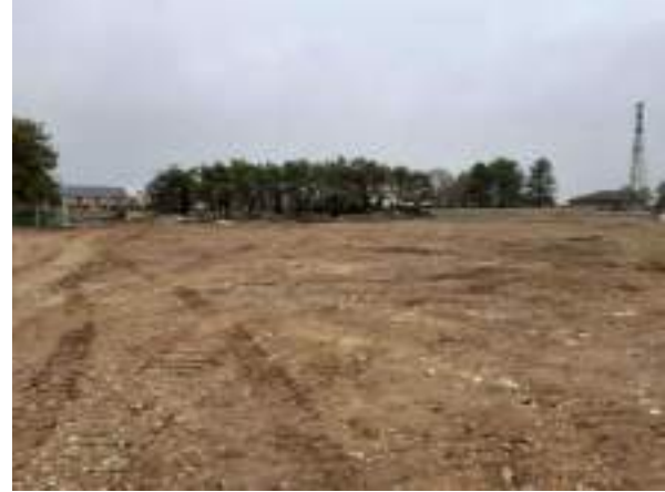
18.10.22 – View southwest across western part of site; topsoil strip carried out prior to site visit.
