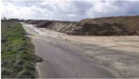
24.03.23 – Stockpiles of contaminated soils located within holding area in wider Heyford development site (5/5).
