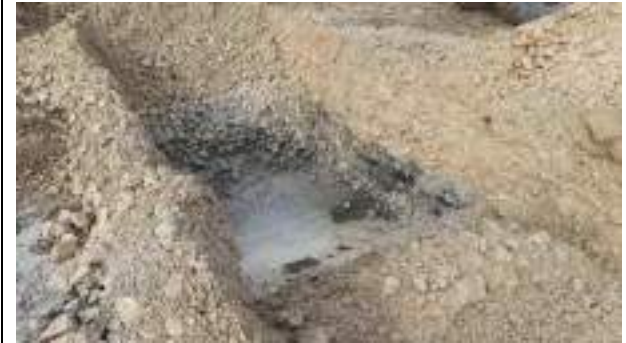
24.03.23 – Excavation progressed to west and thin band of contaminated gravel and clay removed; significant contamination indicators absent from base but still present along northern sidewall – not progressed further as outside proposed of development area.
