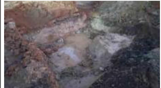
08.12.22 – Cell 7: Excavation progressed eastwards and more significant contamination indicators encountered (Cell 7 Hotspot) so soils were removed down to clean clays; contamination indicators absent from base and western / southern sidewalls but still present in northern and eastern sidewalls.
