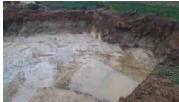
30.11.22 – Cell 2: Excavation progressed northwards and eastwards with contaminated soils removed down to clean clays; contamination indicators still present along southern sidewall.
