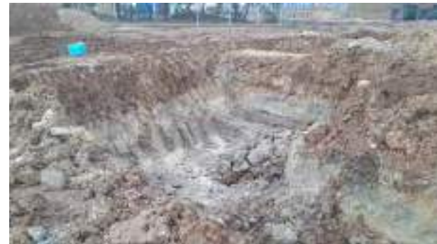
01.02.23 – Excavation continued along eastern extent until significant contamination indicators were no longer present along eastern sidewall (1/2).
