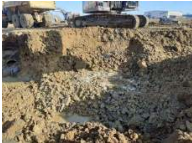
08.02.23 – Cell 6: Excavation of contaminated soils down to bedrock; significant contamination indicators absent along southern sidewall but still present along eastern sidewall.
