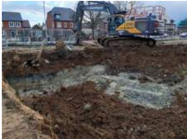
14.03.23 – Cell 9: Excavation progressed southwards with contaminated soils removed down to clean clays; contamination indicators still present in southern sidewall (haul road to be temporarily retained) and western sidewall (unable to progress due to standoff from live drain).
