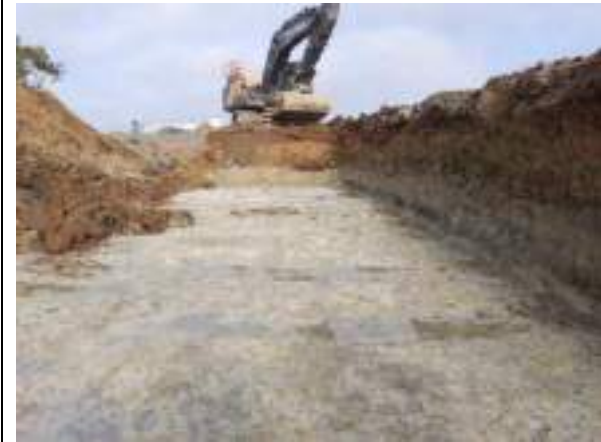
13.02.23 – Cell 8: Excavation progressed northwards with contaminated soils removed down to bedrock; significant contamination indicators absent along eastern sidewall.
