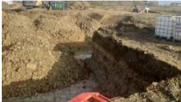
15.02.23 – Cell 8: Excavation progressed northwards / eastwards with contaminated soils removed down to bedrock and clean overburden soils placed into previous excavation area; significant contamination indicators absent along eastern sidewall.
