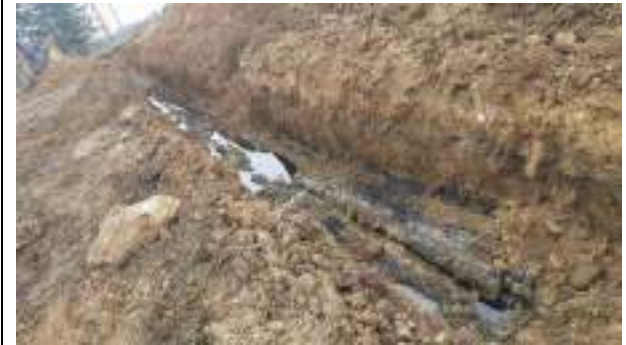
15.03.23 – Cell 10: Relict POL pipeline cut which had not been properly decommissioned; small volume of residual jet fuel (kerosene) leaked into trench.
