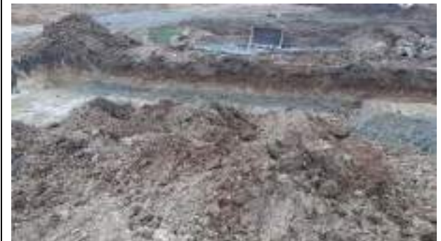
06.03.23 – Contamination indicators still present along western (with exception of the southernmost area) and northern sidewalls.
