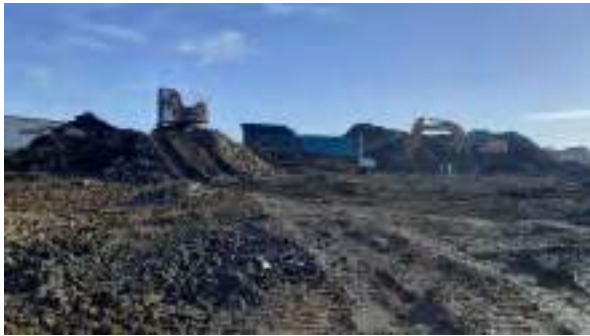
19.01.22 – Crushing of site-recovered hard materials to produce aggregate for reuse on site.
