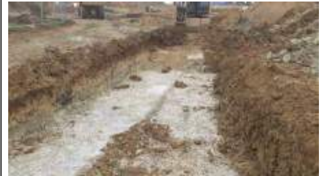
16.02.23 – Cell 9: Excavation progressed eastwards with contaminated soils removed down to bedrock; significant contamination indicators absent along eastern sidewall.
