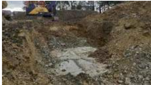
10.02.23 – Cell 7: Excavation progressed southwards with contaminated soils removed down to bedrock; significant contamination indicators absent along eastern and western sidewalls.
