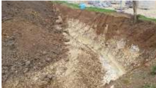
28.02.23 – View along northern extent of eastern NHS excavation area; no contamination indicators present along sidewall.
