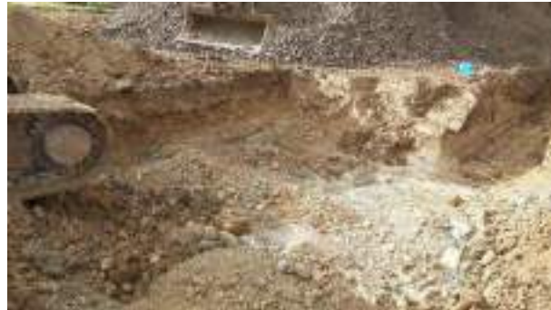
01.03.23 – Southwest corner of SHS excavation area: contaminated soils removed down to bedrock; no significant contamination indicators present along western or southern sidewalls.
