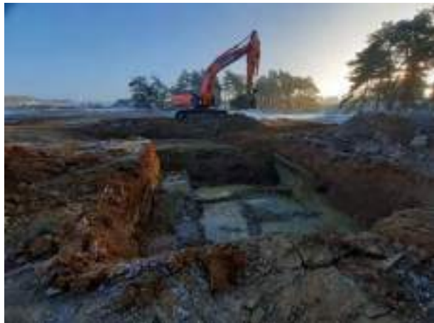
14.12.22 – Cell 8: Excavation of contaminated soils complete; significant contamination indicators absent along northern, southern and western sidewalls.
