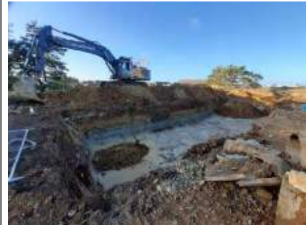
30.01.23 – Cell 2: Excavation progressed northwards until joined with Cell 1 with contaminated soils removed down to bedrock; contamination indicators still present along eastern and western sidewalls.
