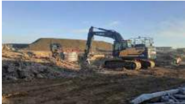
07.12.22 – Location of POL2 (North) tanks.
