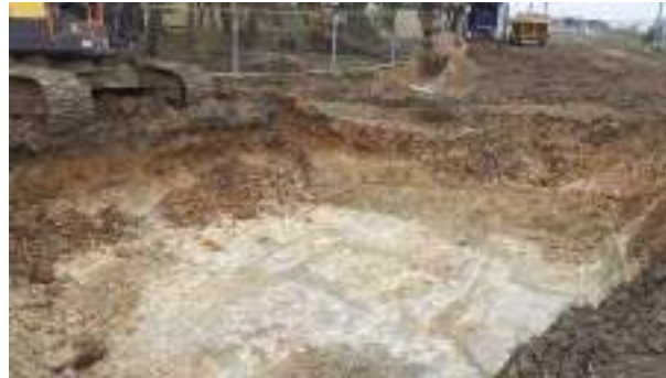
27.01.23 – Cell 1: Excavation progressed northwards with contaminated soils removed down to bedrock and clean overburden soils replaced into excavation; significant contamination indicators absent along western sidewall and western part of northern sidewall.
