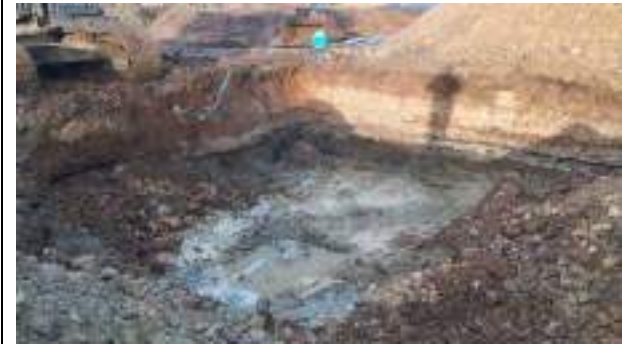
26.01.23 – Impacted soils removed with no significant contamination indicators at base; thin band of impacted soils in northern sidewall but excavation constrained by presence of stockpile.
