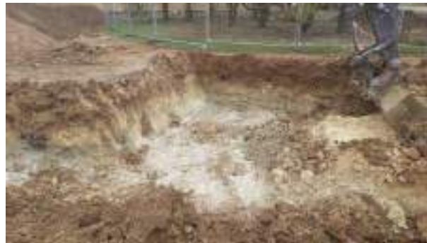
16.02.23 – Cell 9: Excavation progressed eastwards with contaminated soils removed down to bedrock and clean overburden placed into previous excavation area; significant contamination indicators absent along western sidewall.
