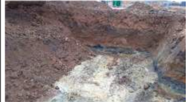
23.03.23 – Cell 13: Excavation progressed westwards with contaminated soils removed down to clean clays; slight contamination indicators still present in eastern sidewall (unable to progress due to live drain) and northern sidewall however these were present at depth (>1.5m bgl) within a thin band of soils (circa. 0.5m thick) so deemed impractical to remove and considered unlikely to present a significant risk to human health and/or the environment.
