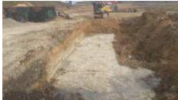
15.02.23 – Cell 8: Excavation progressed northwards / eastwards with contaminated soils removed down to bedrock and clean overburden soils placed into previous excavation area; significant contamination indicators absent along eastern and northern sidewalls.
