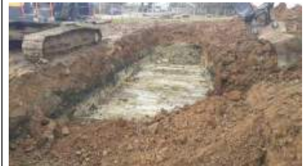
16.03.23 – Cell 9: Excavation progressed westwards with contaminated soils removed down to clean clays and clean overburden soils replaced into excavation; contamination indicators present in all 4 sidewalls so excavation to continue in all directions with exception of eastwards due to presence of live drain.
