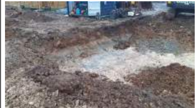
08.03.23 – Excavation progressed northwards / eastwards with contaminated soils removed down to bedrock and clean overburden soils replaced into excavation; thin band of potentially contaminated soil still present along eastern sidewall from ~1.2m bgl however excavation nearing site boundary and any retained impacted soils will be located in future POS area.
