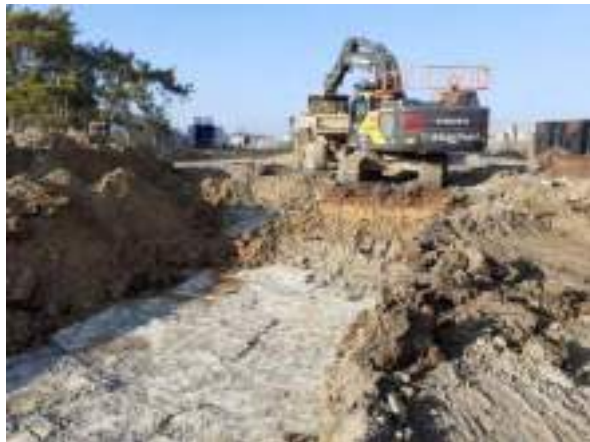
14.02.23 – Cell 8: Excavation progressed northwards with contaminated soils removed down to bedrock and clean overburden soils placed into Cell 2 excavation area; significant contamination indicators absent along eastern sidewall.
