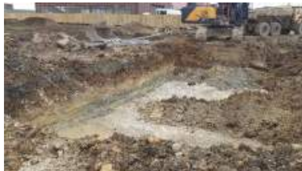
06.03.23 – Excavation continued to west and progressed northwards; contaminated soils removed down to bedrock and clean overburden soils replaced into excavation.
