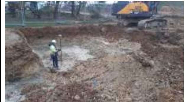
16.02.23 – Cell 9: Excavation progressed eastwards with contaminated soils removed down to bedrock and clean overburden placed into previous excavation area; significant contamination indicators absent along eastern sidewall.
