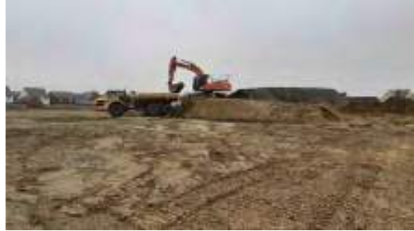
20.02.23 – Removal of contaminated soils to holding area within wider Heyford development site.
