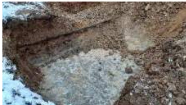
12.12.22 – Contaminated soils underlying relict pipeline removed down to bedrock; contaminated soils present along all four sidewalls near excavation base.
