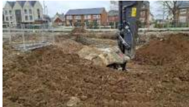
23.03.23 – Cell 13: Commencement of excavation from north of Cell 10 / west of live drain.
