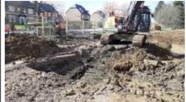
22.03.23 – Cell 12: Commencement of excavation from south of Cell 9 / west of live drain.
