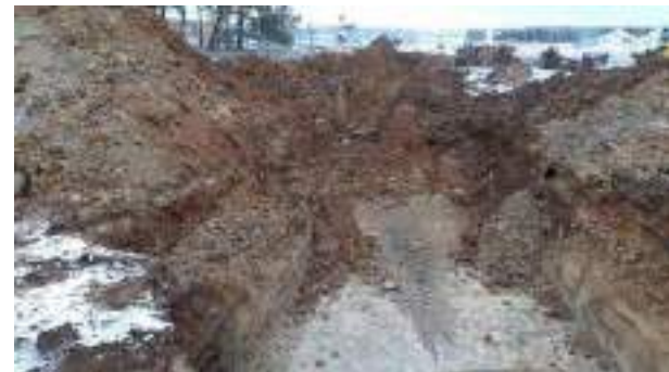
12.12.22 – Relict pipeline removed but excavation of contaminated soils paused until later date.
