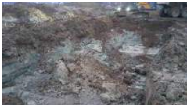
01.02.23 – Excavation continued along eastern extent until significant contamination indicators were no longer present along eastern sidewall (2/2).
