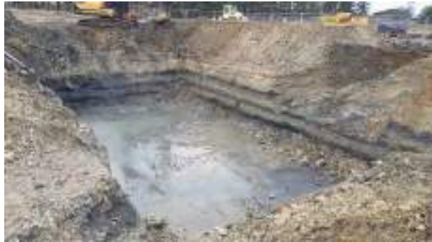
11.01.23 – POL2 (North) tanks removed and base and sidewalls exposed (partially limestone bedrock); view southwest.
