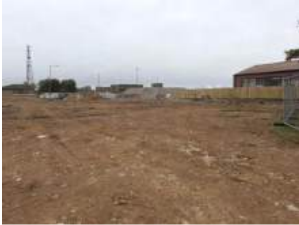
18.10.22 – View west across northern part of western part of site; topsoil strip carried out prior to site visit.
