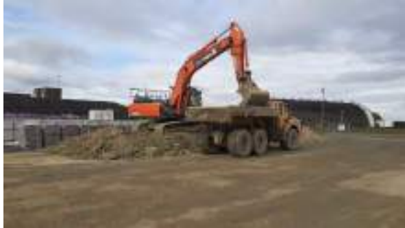
07.03.23 – Removal of contaminated soils to holding area within wider Heyford development site.
