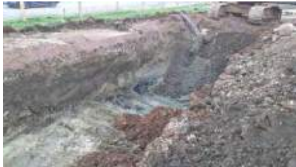
22.03.23 – Cell 12: Excavation progressed westwards with contaminated soils removed down to clean clays; contamination indicators present in southern sidewall but unable to progress due to standoff from Camp Road / live services.
