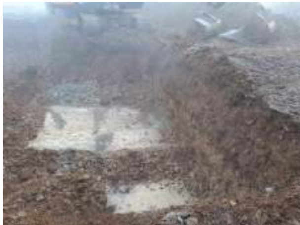
08.02.23 – Cell 5: Excavation progressed to south and east with contaminated soils removed down to bedrock.
