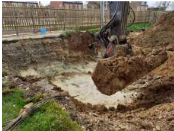
05.12.22 – Cell 3: Commencement of excavation to east of southern part of Cell 2; contamination indicators still present along southern sidewall.
