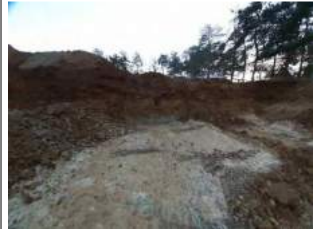
06.02.23 – Cell 5: Excavation progressed to south and east with contaminated soils removed down to bedrock.
