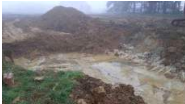
01.12.22 – Cell 2: Excavation progressed northwards (until joined with Cell 1) and eastwards with contaminated soils removed down to clean clays.
