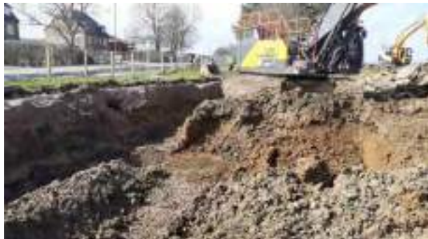
23.03.23 – Cell 12: Excavation continued to the north of previous excavation area / west of Cell 9.
