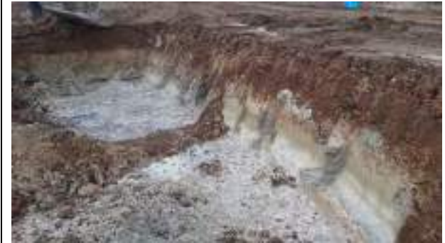
01.02.23 – Cell 3: Contamination indicators present along northern sidewall.
