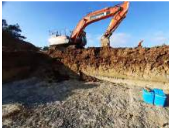
01.02.23 – Cell 2: Excavation progressed westwards and northwards with contaminated soils removed down to bedrock; significant contamination indicators absent along western and southern sidewalls.
