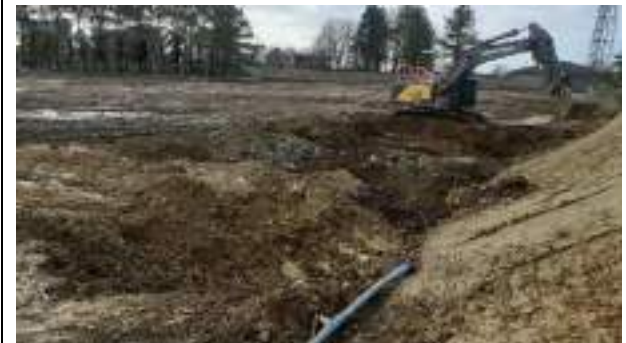
26.01.23 – View of hotspot area excavated over the previous 2 days during backfilling with retained overburden soils.
