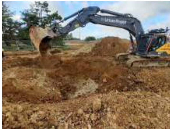
31.01.23 – Cell 2: Excavation continued to west of previous excavation area (southwest corner of Cell 2) and progressed northwards with contaminated soils removed down to bedrock; significant contamination indicators absent along western sidewall.
