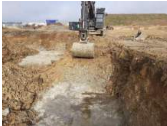
14.02.23 – Cell 8: Excavation progressed northwards with contaminated soils removed down to bedrock and clean overburden soils placed into Cell 2 excavation area; significant contamination indicators absent along eastern sidewall.
