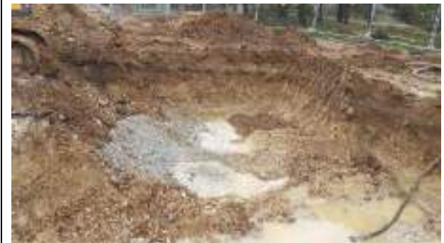
02.02.23 – Cell 4: Excavation progressed southwards from southwest corner of Cell 3 with contaminated soils removed down to bedrock; significant contamination indicators absent along western sidewall but still present along southern sidewall.
