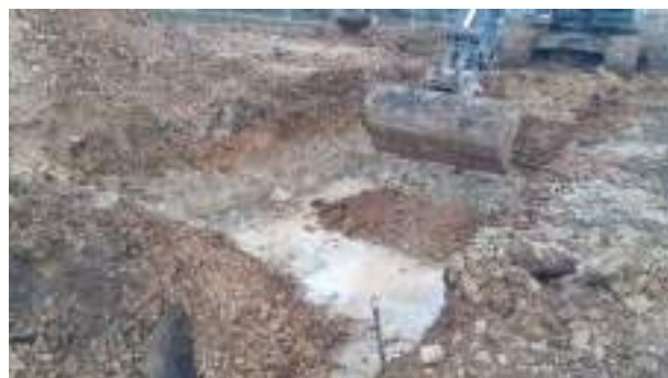
26.01.23 – Cell 1: Excavation progressed northwards with contaminated soils removed down to bedrock and clean overburden soils replaced into excavation; significant indicators of contamination absent along western sidewall.
