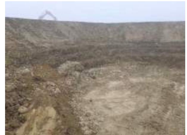
14.11.22 – View west along northern edge of POL21A area following breakout and removal of tank.
