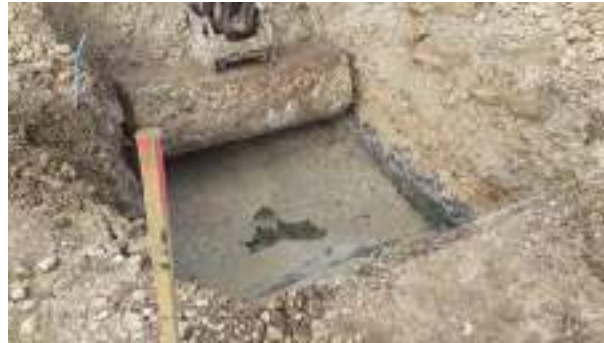
24.03.23 – Thin band of contaminated gravel and clay removed; significant contamination indicators absent from base but still present along northern sidewall – not progressed any further as outside of proposed development area (i.e. outside of future plot footprints and gardens).
