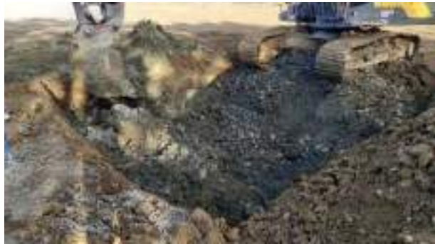
08.12.22 – Cell 6: Soils demonstrating slight contamination indicators but not significant enough to warrant removal so excavated, aerated and replaced into excavation.
