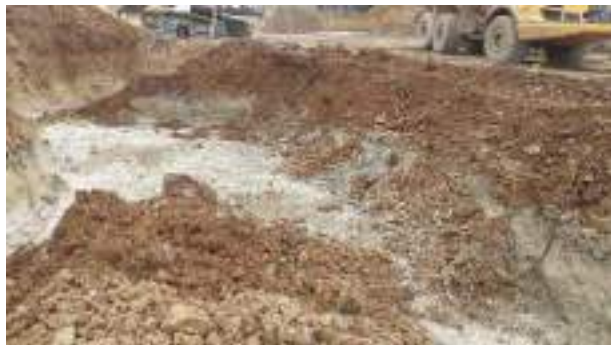
21.02.23 – Excavation progressed southwards alongside access road which curves to the east with contaminated soils removed down to bedrock and clean overburden soils replaced into excavation area; contaminated soils continued beneath roadway (1/2).
