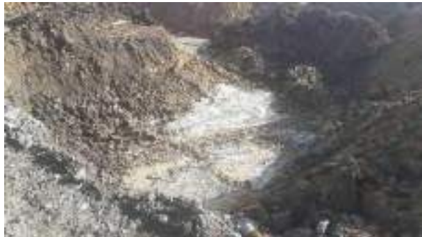
15.02.23 – Cell 8: Excavation progressed northwards / eastwards with contaminated soils removed down to bedrock and clean overburden soils placed into previous excavation area.
