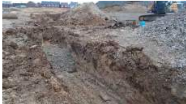
01.03.23 – Contaminated soils encountered at ~1.3m bgl during removal of relict POL pipeline.
