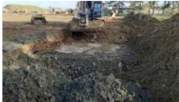
08.12.22 – Cell 6: Excavation progressed eastwards and more significant contamination indicators encountered (Cell 6 Hotspot).
