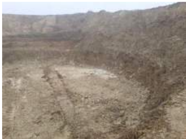
14.11.22 – View west along southern edge of POL21A area following breakout and removal of tank.
