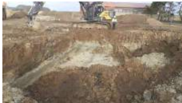
02.02.23 – Excavation continued along western extent until significant contamination indicators were no longer present in western sidewall.
