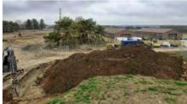
28.02.23 – Relocation of site-recovered topsoil stockpiles from centre-northwest of site (stockpile refs: TS-SP3 & TS-SP4) to north of site for future placement within northern POS area.
