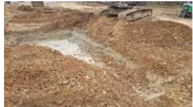
21.02.23 – Excavation progressed southwards with contaminated soils removed down to clean clays / solid bedrock; contamination indicators not present along northern part of western sidewall (~7m) but were as excavation continued southwards.
