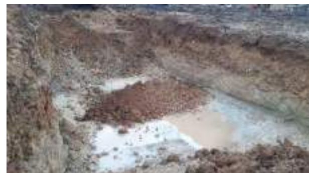
26.01.23 – Cell 1: Excavation progressed northwards with contaminated soils removed down to bedrock and clean overburden soils replaced into excavation; contamination indicators still present along eastern sidewall.
