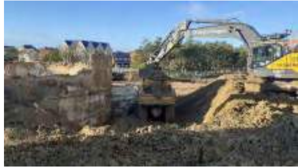
22.11.22 – Excavation of soils around POL21C tank to fully expose walls; soils demonstrating contamination indicators removed to contamination stockpiles in northwest.
