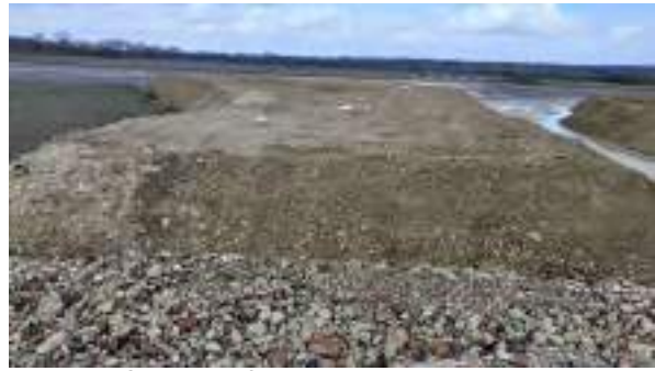
24.03.23 – Stockpiles of contaminated soils located within holding area in wider Heyford development site (2/5).
