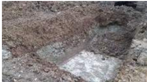
01.02.23 – Starting point of excavation; indicators of contamination present in all sidewalls underlying clean overburden; contaminated soils excavated to bedrock.
