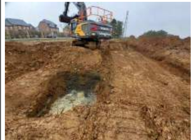
20.03.23 – Cell 10: Excavation continued to south of previous excavation area towards northern extent of Cell 9.
