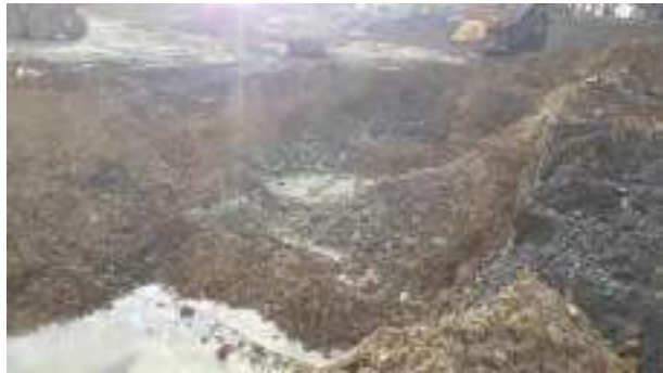
10.02.23 – Cell 7: Excavation progressed northwards with contaminated soils removed down to bedrock; significant contamination indicators absent along eastern sidewall.
