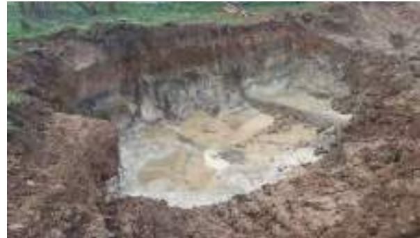
30.11.22 – Cell 2: Commencement of excavation to southwest of demolished interceptor (southwest corner of Cell 2).
