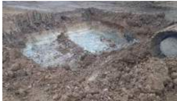
16.02.23 – Cell 9: Contaminated soils removed down to bedrock; significant contamination indicators absent along western sidewall.
