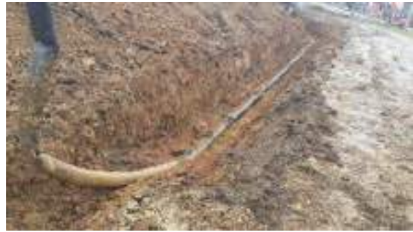
15.03.23 – Second POL pipeline uncovered in southwest of site – no evidence of leakage (1/2).
