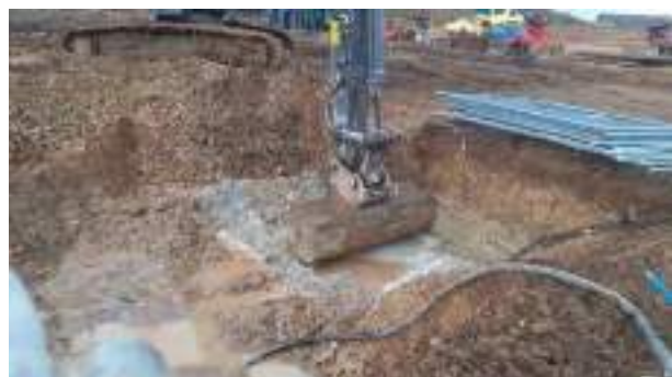
26.01.23 – Cell 1: Excavation progressed to east of previous excavation area up unto haul road (which was to be temporarily retained) with contaminated soils removed down to bedrock; contamination indicators still present along eastern sidewall.
