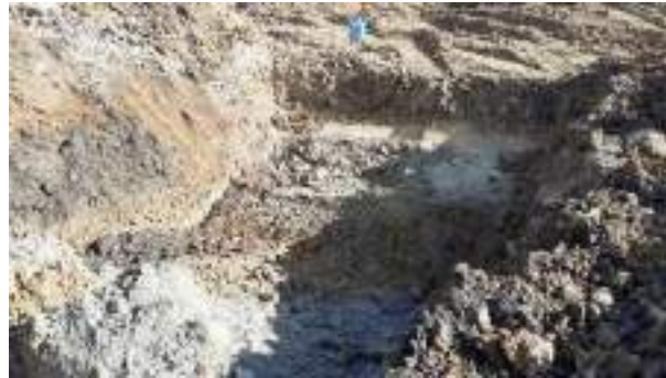
02.03.23 – No contamination indicators present along southern sidewall of excavation along former roadway.
