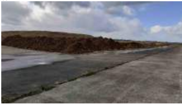
24.03.23 – Stockpiles of contaminated soils located within holding area in wider Heyford development site (3/5).
