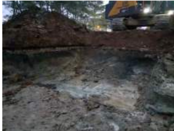
13.12.22 – Cell 8: Excavation progressed westwards with contaminated soils removed down to clean clays; significant contamination indicators absent along northern and southern sidewalls.
