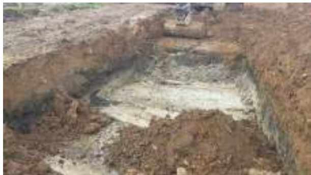
16.03.23 – Cell 9: Excavation progressed westwards with contaminated soils removed down to clean clays.
