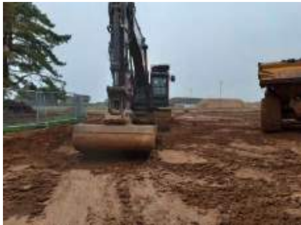
29.11.22 – Cell 1: Commencement of excavation in vicinity of former “Valve Pit” (southwest corner of Cell 1).
