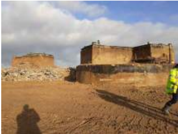
08.11.22 – Upper extents of POL21B & POL21C tanks exposed and commencement of demolition (POL21C only).
