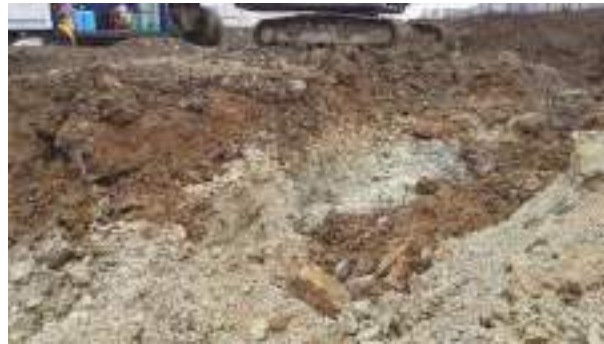
08.03.23 – Excavation progressed eastwards with contaminated soils removed down to bedrock and clean overburden soils replaced into excavation; significant contamination indicators absent along northern sidewall.
