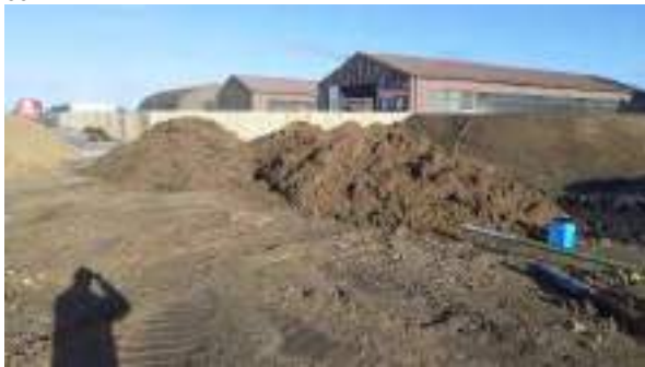
19.01.22 – Small stockpile of topsoil recovered from the area around trial pit 'JTP8' (stockpile ref: TS-SP4) in centre-northwest.
