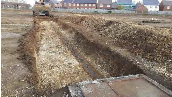
25.10.22 – Exposure of relict POL pipeline crossing central / northern parts of site traversing from southwest to northeast.
