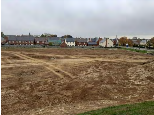
18.10.22 – View southeast across central / southern parts of site; topsoil strip completed in these areas prior to arrival.
