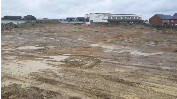
09.11.22 – Earthworks complete: view north across north of site; stockpiles of hardstanding previously located in north of site relocated to wider Phase 10 development area.
