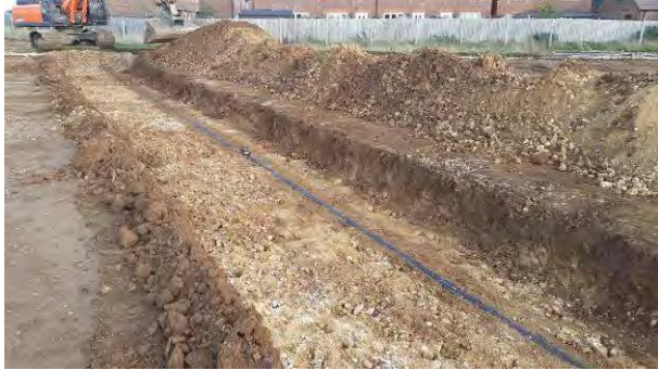
25.10.22 – Continued exposure of relict POL pipeline crossing central / northern parts of site.
