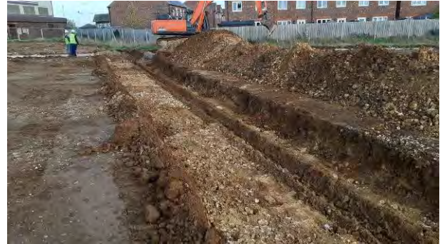
25.10.22 – No contamination indicators in soils underlying eastern section of relict POL pipeline.
