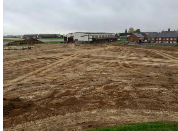
18.10.22 – View northeast across central / north-eastern parts of site; topsoil strip completed in these areas prior to arrival.
