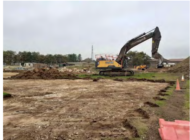
18.10.22 – Final vegetation / topsoil strip being carried out in northwest corner of site.
