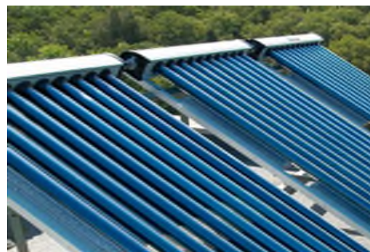
Figure 9: Solar thermal hot water panels.
