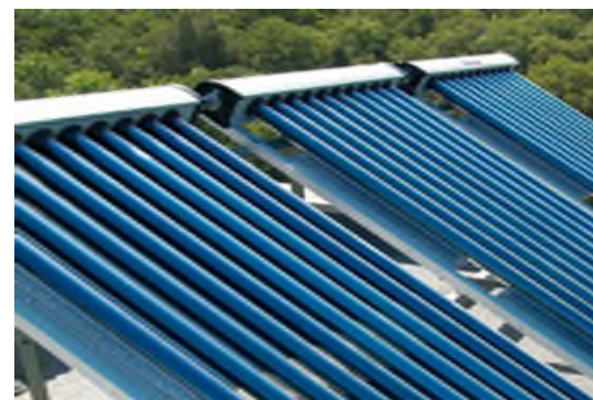
Figure 10: Solar thermal hot water panels.
