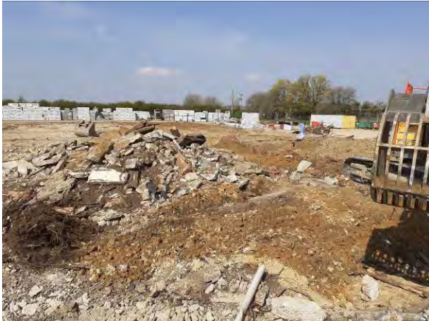
20.04.21 – Handpicking of ACM fragments within localised area in the north (HS-ACM) by specialist sub-contractor
