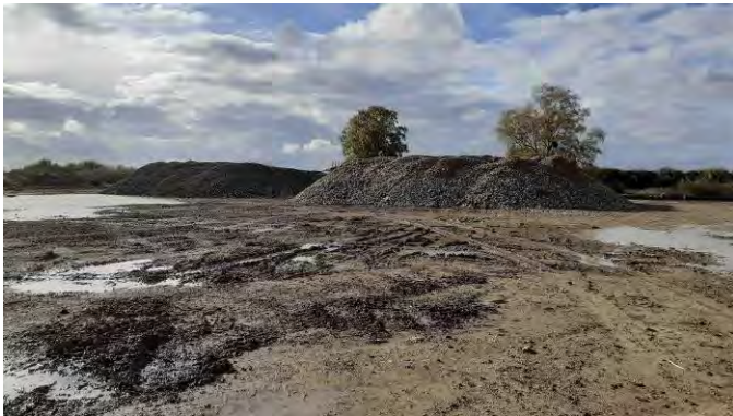
25.10.22 – Stockpiles of site-generated aggregate present along western boundary: Ph9-Agg-4 (left) & Ph9-DH-Agg (right).
