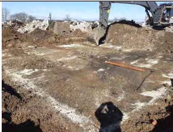
09.03.21 – Tank surface exposed confirming 3 tanks present. Removal of cover confirms water filled with some floating oil product
