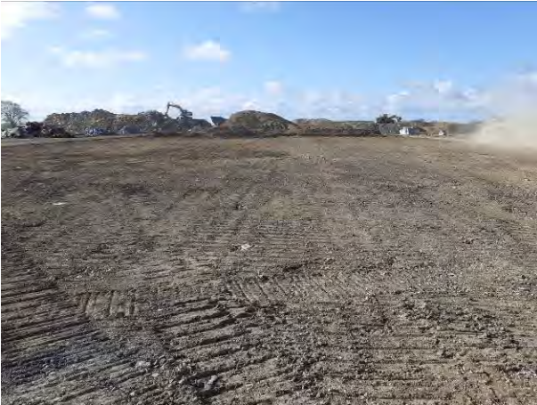
06.04.21 – Western part of site demolition complete, hardstanding removed, and site regraded ahead of formation sampling
