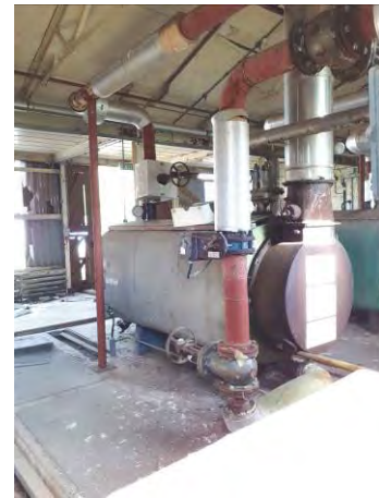
22.05.18 – boilers within boiler house
