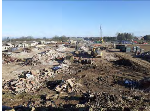
09.03.21 – Building demolition complete in the northern part of the site, recovery of hardstanding for processing
