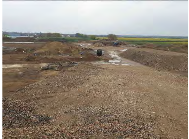
28.04.21 – Eastern view of southern end of site with site-generated aggregate stockpiles present
