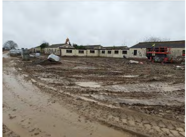
20.01.21 - Asbestos strip in northern buildings
