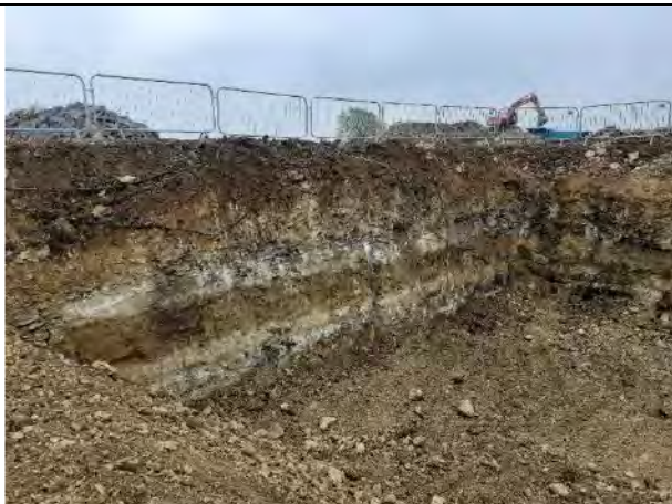
28.04.21 – Base of excavation at approximately 2.8m bgl. Limestone gravel present to 2.3m bgl with limestone bedrock to base
