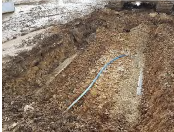
17.02.21 – Excavation of trench to 0.8m due to presence of possible drain and water pipe
