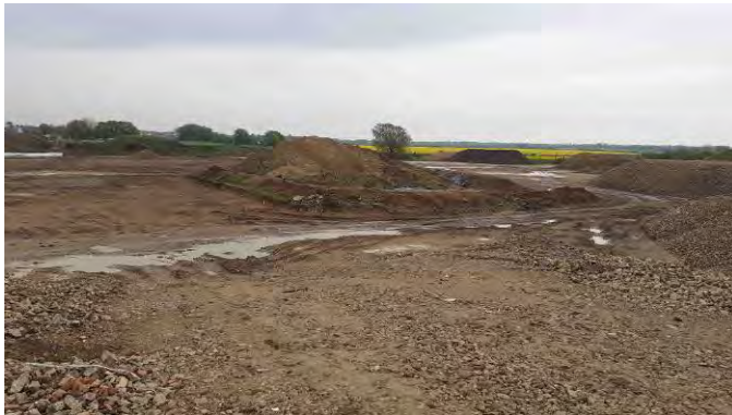
13.05.21 -South-eastern view. Temporary stockpile of contaminated soils from Phase 9 baseball pitch remains within quarantine area
