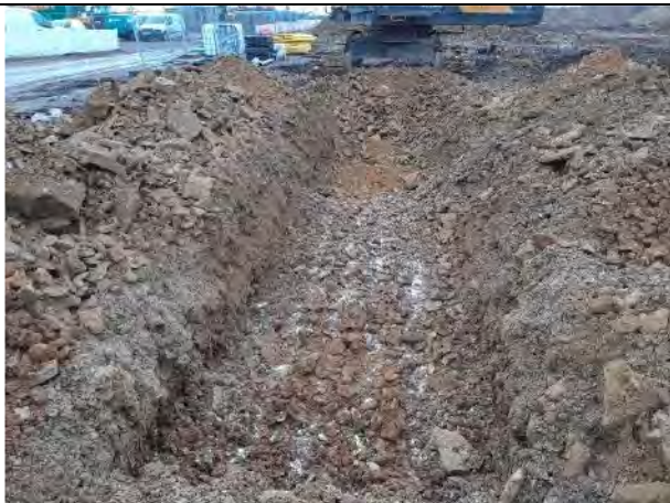
28.04.21 – Trench 2 excavated adjacent to access road into site, no black gravel encountered
