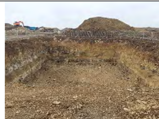
28.04.21 – Excavation void following removal of tanks. Natural soils present on all sides. No evidence of staining on sidewalls or base
