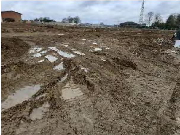
17.02.21 – Location of Hydrock hotspot located by GPS
