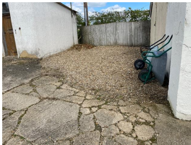
Figure 10. Areas of concrete and gravelled hard-standing to the north-west of the house.
