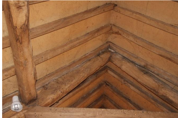
12. Bat droppings coming from gap by rafter/beam
