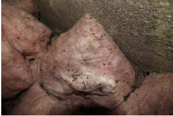
9. Pipistrelle bat droppings next to eastern chimney
