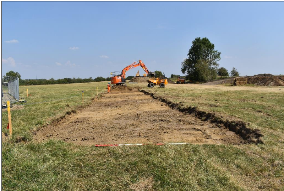
Plate 1: Mid-excitation view of ridge and furrow after topsoil strip adjacent to gas main, looking northeast
