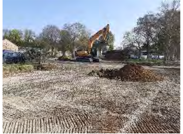
20.04.21 – Excavation of validation pits to verify formation soils in the north of the site.
