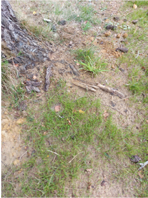
P5. Although evidence of root damage was limited around the base of T34, it suggests that the recent trenching and other groundworks were in close proximity to the stem.
