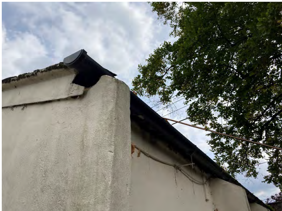
Photograph 12 - Building 2 lifted fascia
