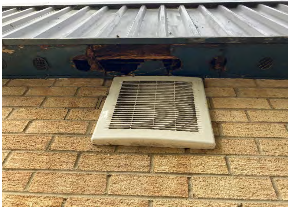
Photograph 9 - Building 1 damaged Soffit
