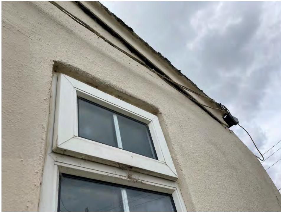
Photograph 11 - Building 2 lifted fascia
