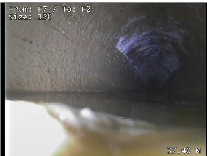
Other attached deposits from 7 to 5 o'clock 5% cross-sectional area loss - Remark Scale, Finished
