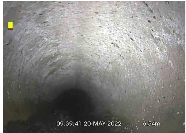
SW9X_bf174e5f-7231-42d9-a190-5e3acabe447a_20220524_153346_311.jpg, 00:00:32, 6.54 m Settled deposits, fine, 10% cross-sectional area loss, start
