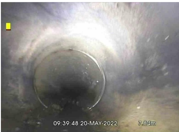
SW9X_09760fb7-84e8-4291-9d2e-5da4e6c0aa3f_20220524_153419_676.jpg, 00:00:39, 7.84 m Junction at 9 o'clock, diameter: 150mm
