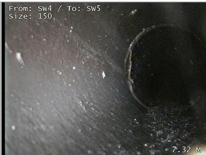
Other settled deposits 5% cross-sectional area loss - Remark: Slit, Start
