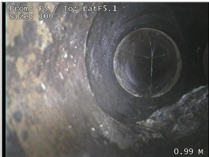
Settled deposits fine 10% cross-sectional area loss, at joint
