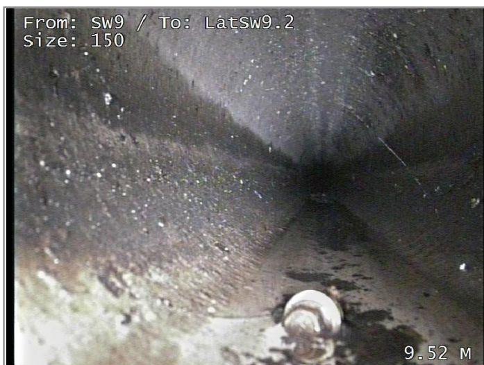
Bolt in pipe
