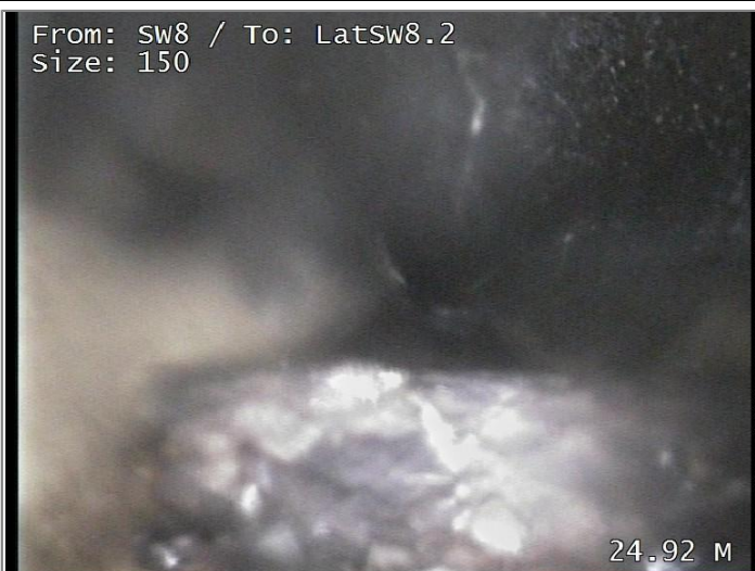
Settled deposits fine 5% cross-sectional area loss
