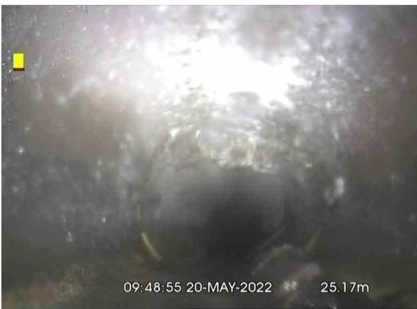
SW8X_4b8631f0-a9bb-4ee2-b759-69b4075cb24a_20220524_154757_309.jpg, 00:01:33, 25.17 m Other obstacles from 4 o'clock to 5 o'clock, 5% cross-sectional area loss
