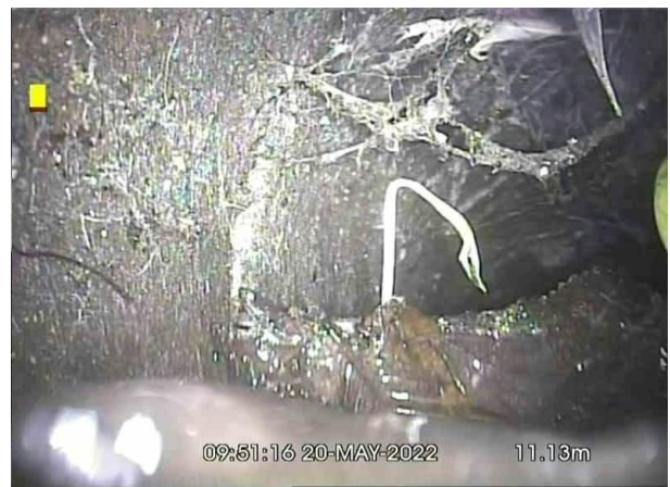
SW8aX_17b95e9e-220e-4be2-a1a7-3f4044087fcb_20220524_155231_647.jpg, 00:00:55, 11.13 m Settled deposits, hard or compacted, 20% cross-sectional area loss, start
