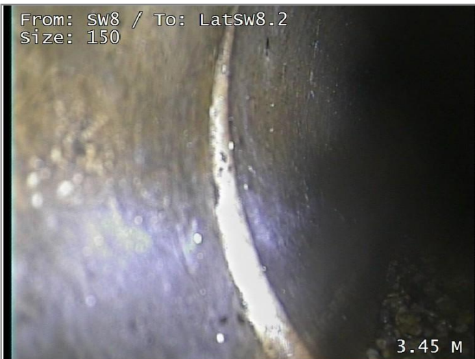
Other settled deposits 5% cross-sectional area loss - Remark: Silt/Stones, Start
