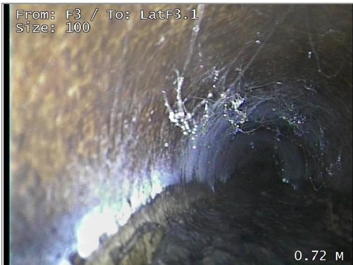
Settled deposits fine 5% cross-sectional area loss, Start
