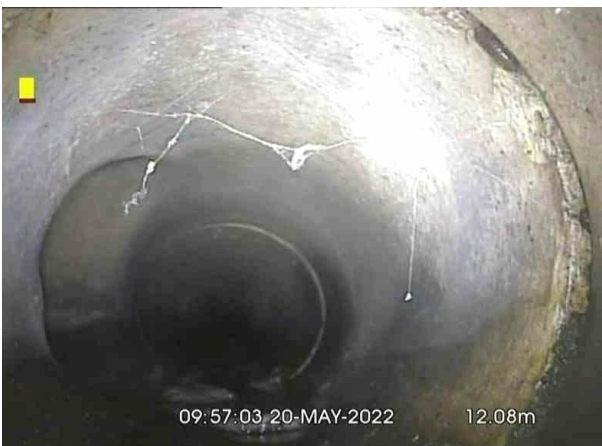
SW7X_dc5a9c8d-b0b0-4b9f-9e3a-5ba773705f6a_20220524_155603_277.jpg, 00:00:41, 12.08 m Junction at 9 o'clock, diameter: 100mm
