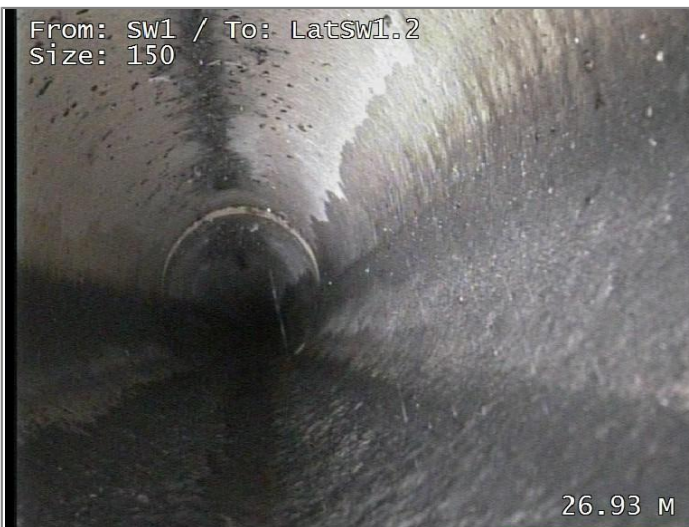
Survey abandoned - Remark: Unable to push further
