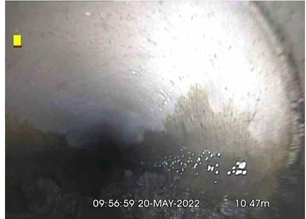
SW7X_dc245387-ccb8-4121-b59f-93122fa6a0b2_20220524_155543_172.jpg, 00:00:36, 10.47 m Settled deposits, fine, 10% cross-sectional area loss, start
