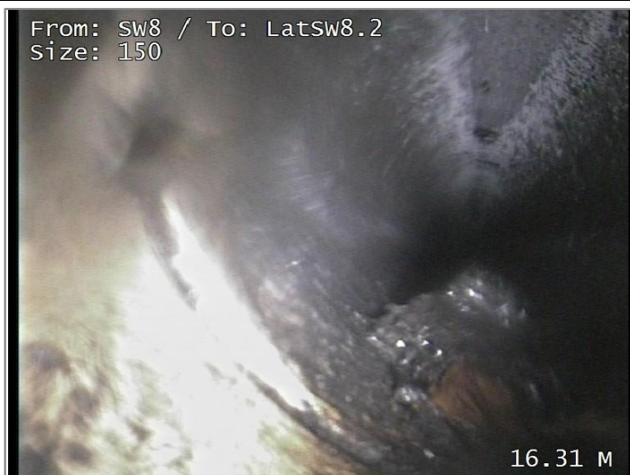
Other settled deposits 5% cross-sectional area loss - Remark: Silt
