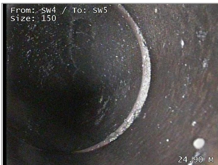
Survey abandoned - Remark: Unable To Push Further
