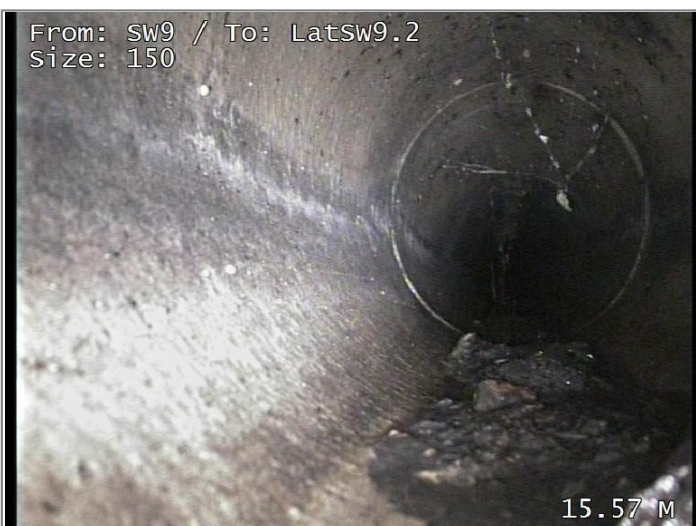
Settled deposits fine 5% cross-sectional area loss, Start
