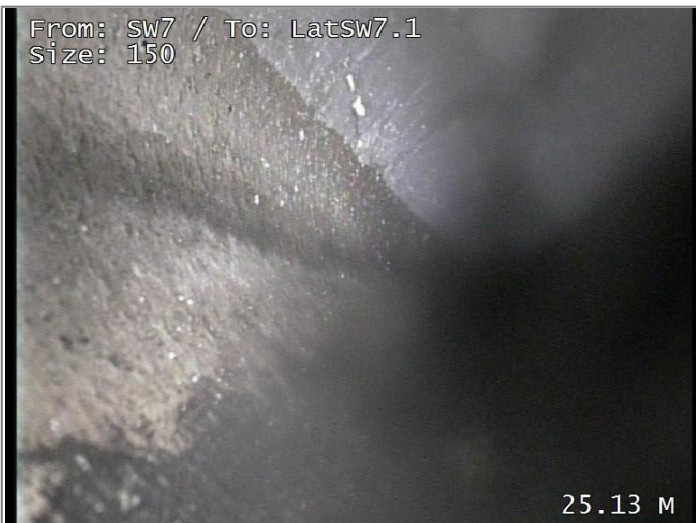
Other settled deposits 10% cross-sectional area loss - Remark: Slit, Finished
