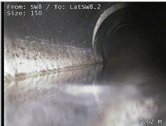
Other settled deposits 5% cross-sectional area loss - Remark: Silt/Stones, Finished
