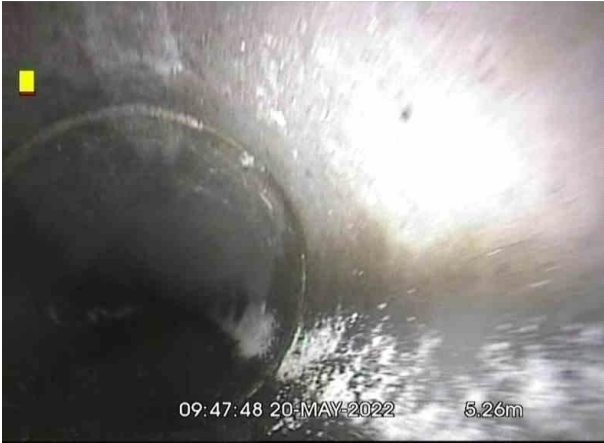
SW8X_4f221960-a994-46da-b7d0-640ef9967412_20220524_154449_738.jpg, 00:00:27, 8.57 m Junction at 10 o'clock, diameter: 150mm
