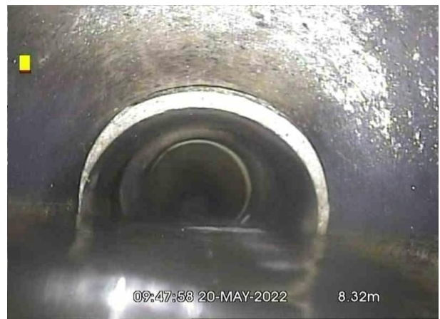
SW8X_e9f3c9bc-7f79-452e-9013-7e3c0039f48b_20220524_154353_069.jpg, 00:00:36, 8.32 m Joint displaced, medium
