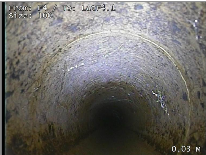
Crack circumferential from 9 to 5 o'clock
