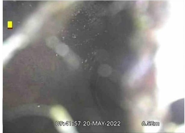
SW9aX_25ac594d-fd63-472f-92d9-7faca6f72f29_20220524_153818_334.jpg, 00:00:41, 6.19 m Loss of vision, other, obscured by cobwebs
