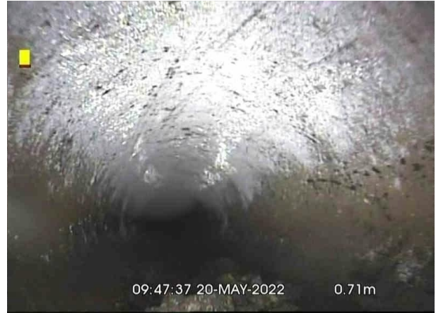
SW8X_4007ea33-9ca3-47e4-84b9-524f0be99d4e_20220524_154241_227.jpg, 00:00:15, 0.51 m Settled deposits, fine, 10% cross-sectional area loss, start
