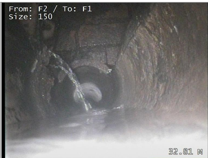
Water level throughout pipe work due to constant flow
