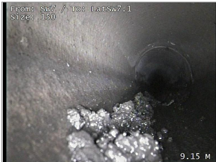
Other settled deposits 10% cross-sectional area loss - Remark: Slit, Start
