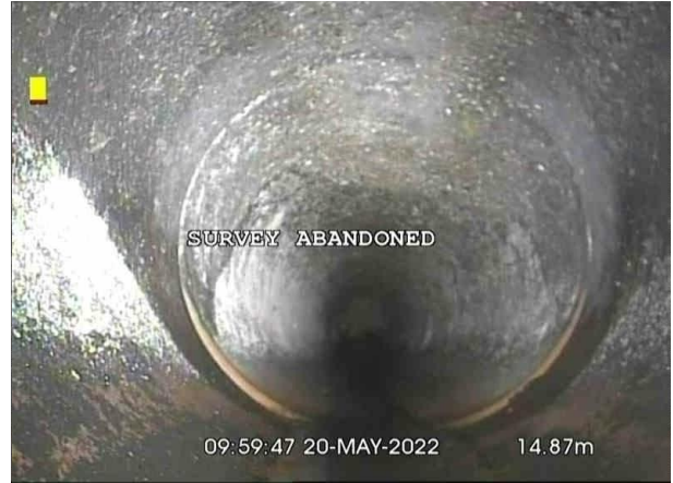
SW7aX_5a3407ad-2d90-450c-9c57-37b4580906bc_20220524_160033_913.jpg, 00:01:01, 14.70 m Survey abandoned, Out Off Cable
