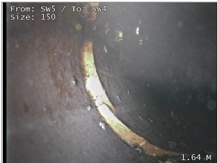
Broken pipe at 8 o'clock, at joint
