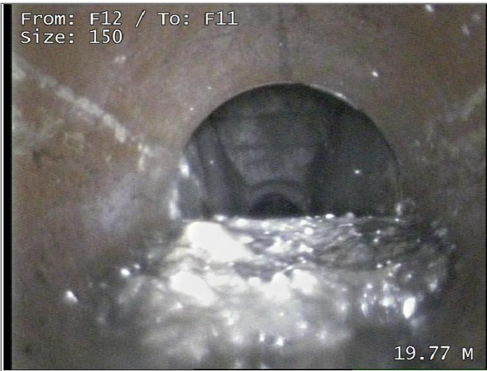
Other attached deposits from 8 to 4 o'clock 25% cross-sectional area loss - Remark Scale
