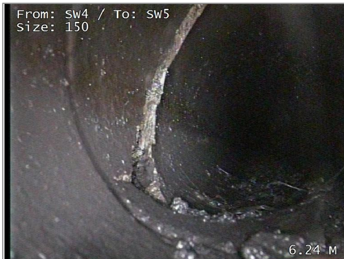
Broken pipe at 7 o'clock, at joint
