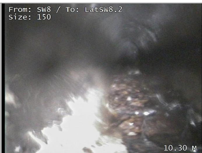
Settled deposits fine 5% cross-sectional area loss, Start
