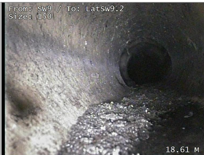
Settled deposits fine 5% cross-sectional area loss, Start
