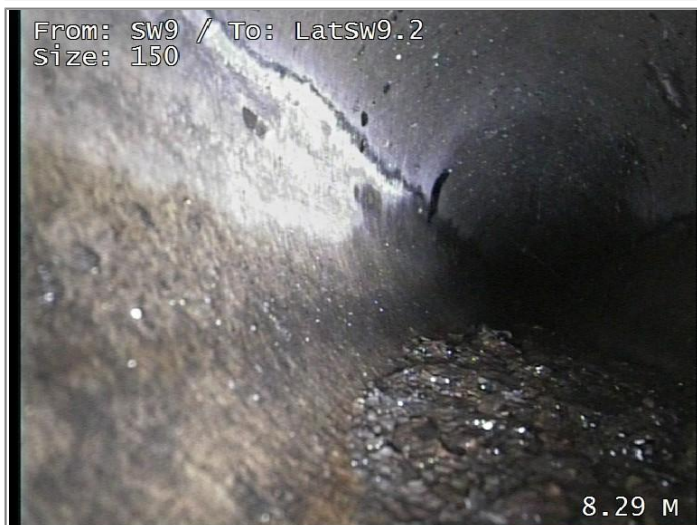
Settled deposits fine 10% cross-sectional area loss, Start
