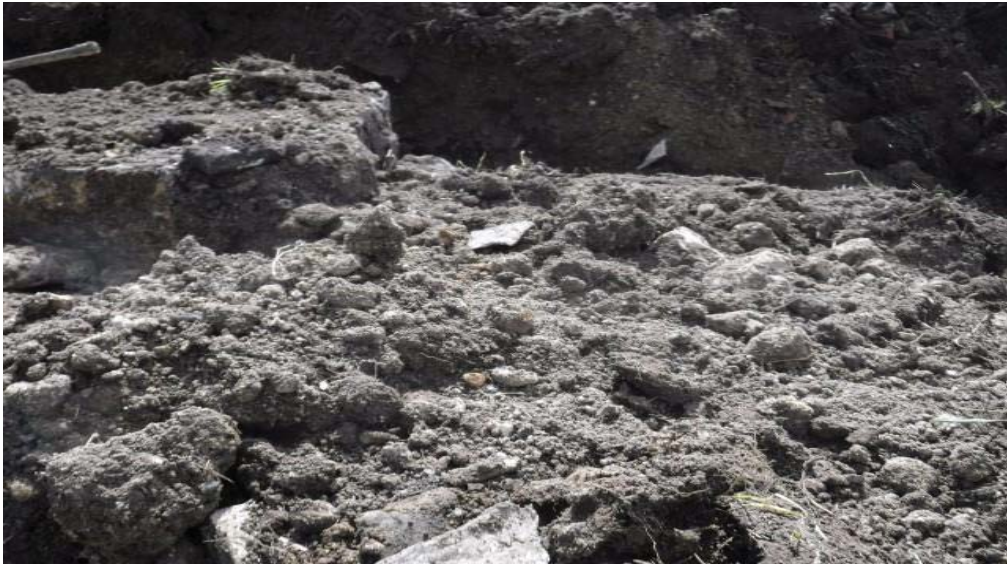
Suspected ACM - Trial Trench TP16
