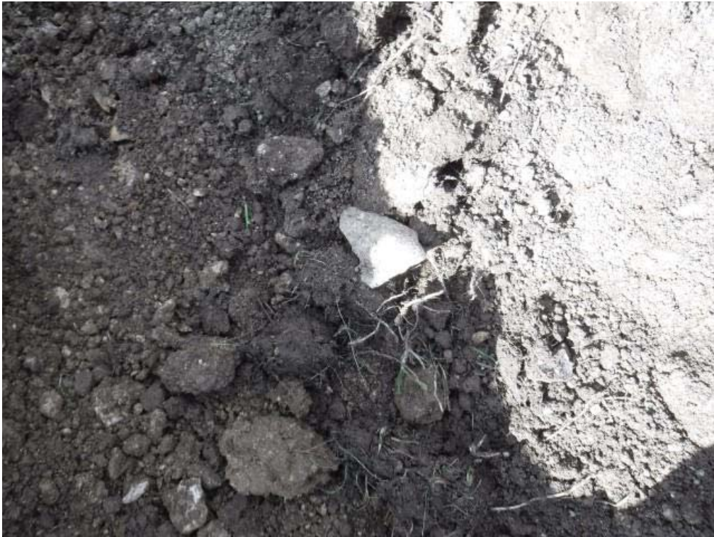
Suspected ACM - Trial Trench TP15
