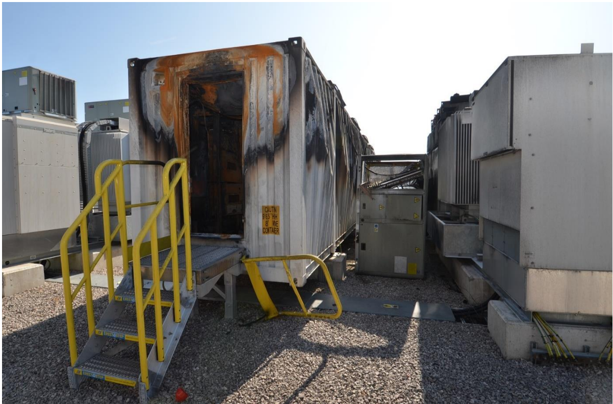
Image above: Exterior of unit with pressure damage to side.
