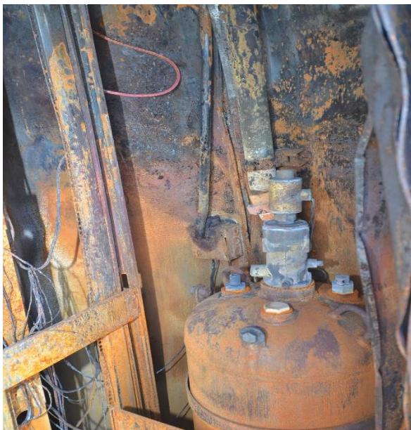
Image below left: Fire damaged NOVEC 1230 unit.
