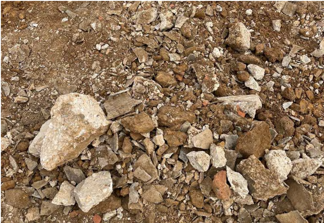
Plate 2: Asbestos cement fragments through the near surface hardcore sub-base to slab.
