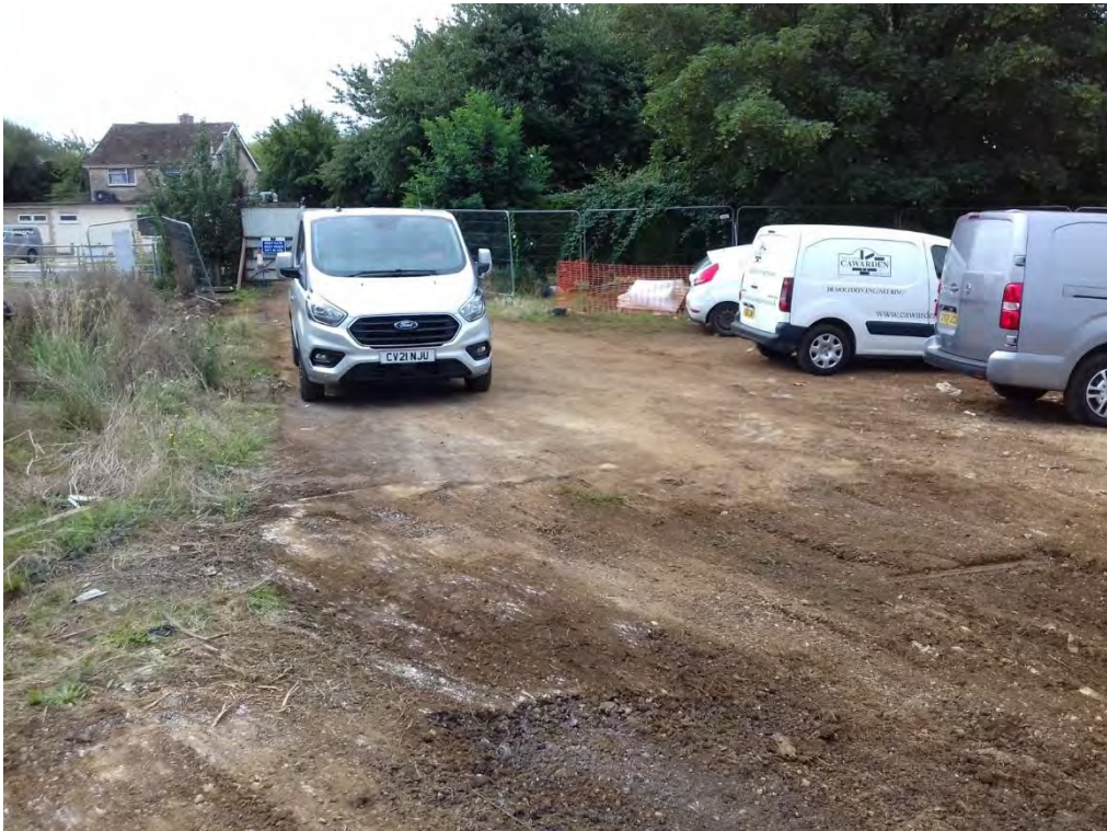
Plate 5: Hardcore layer chased out to access road entrance. (Face 1 sample taken from this location).
