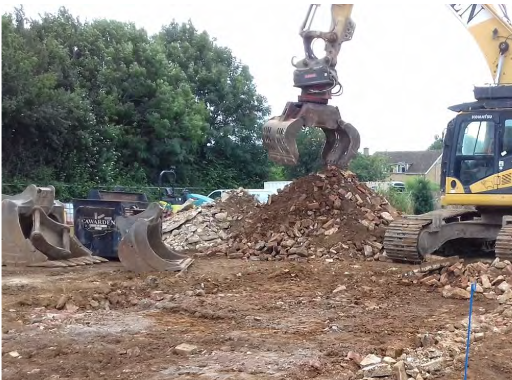
Plate 6: Stockpile of asbestos contaminated soils and concrete for off-site disposal.
