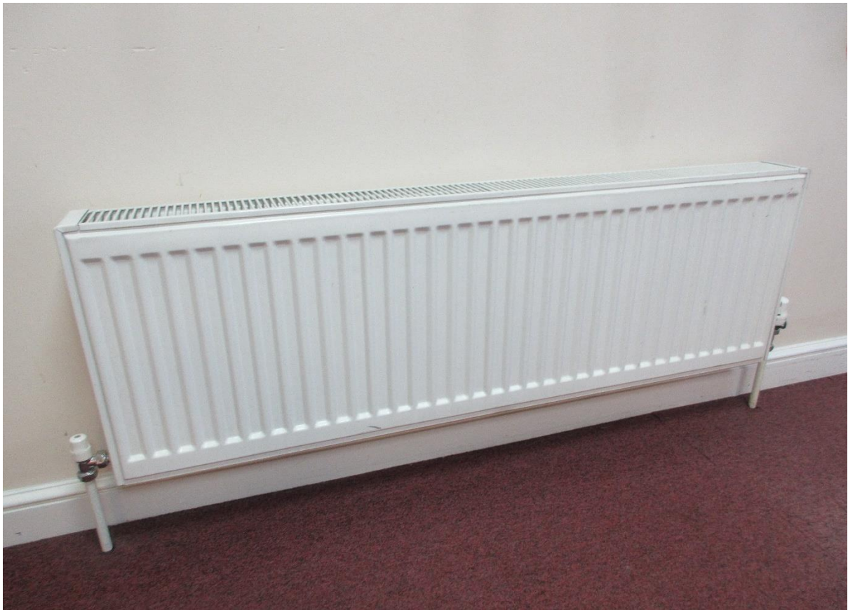
Standard radiator heating
