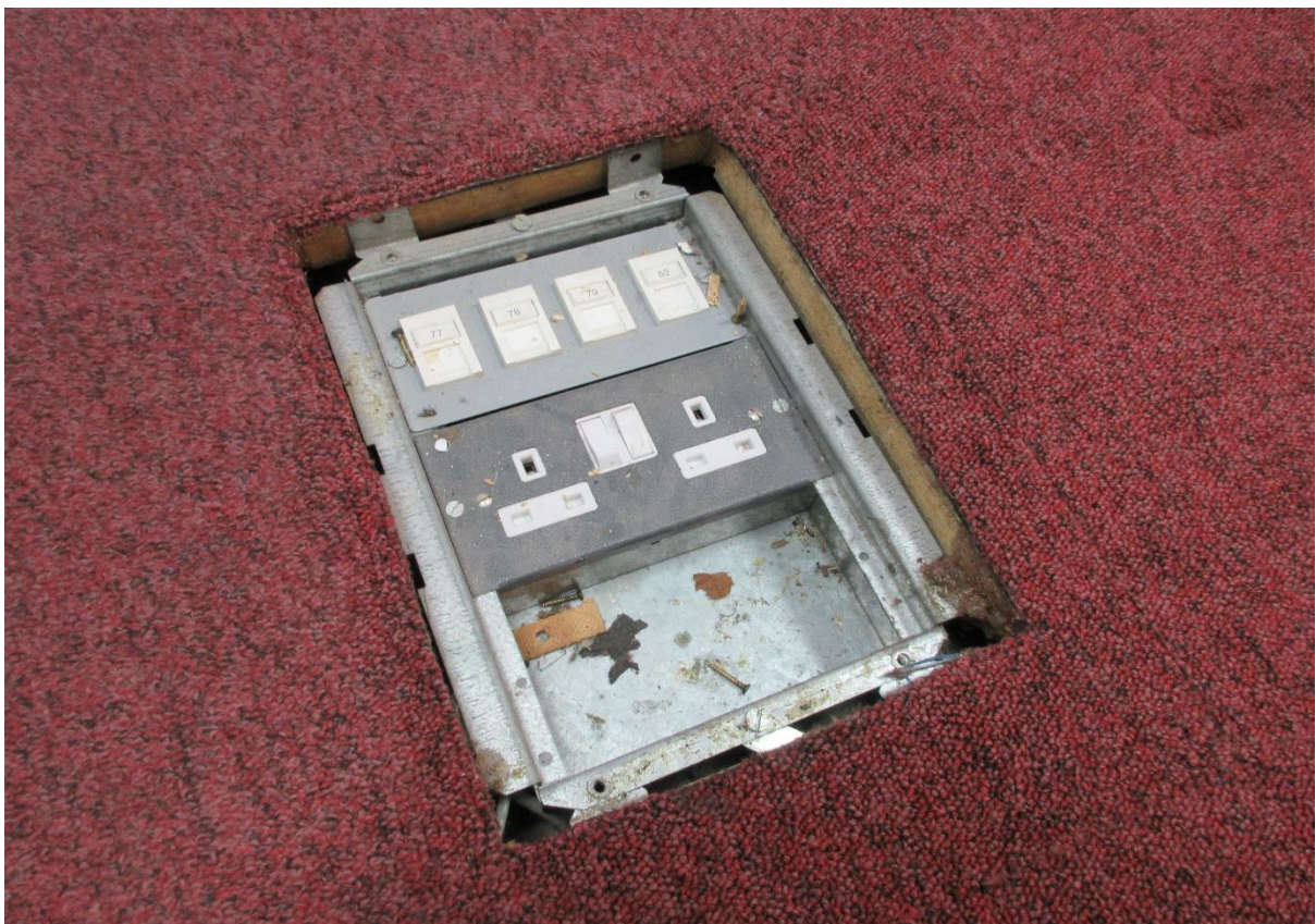
Typical floor box
