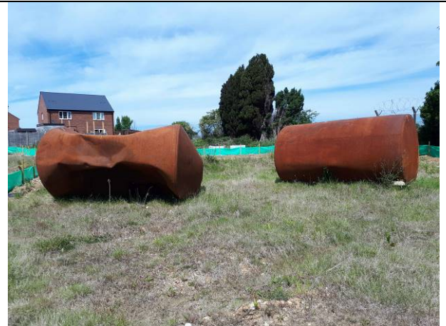
02.06.20 – Removed USTs as part of remedial works awaiting off-site removal for recycling
