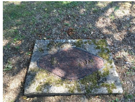
FIGURE 10: EXISTING KLARGESTER UTILISED FOR FOUL WATER
